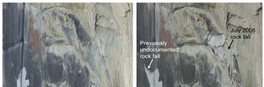
Figure 5. Gigapixel panoramic photograph of the northwest face of Half Dome from the Diving Board (top), white rectangle shows location of lower views of the face prior to (left) and after (right) rock falls occurring between 2005 and 2006.
