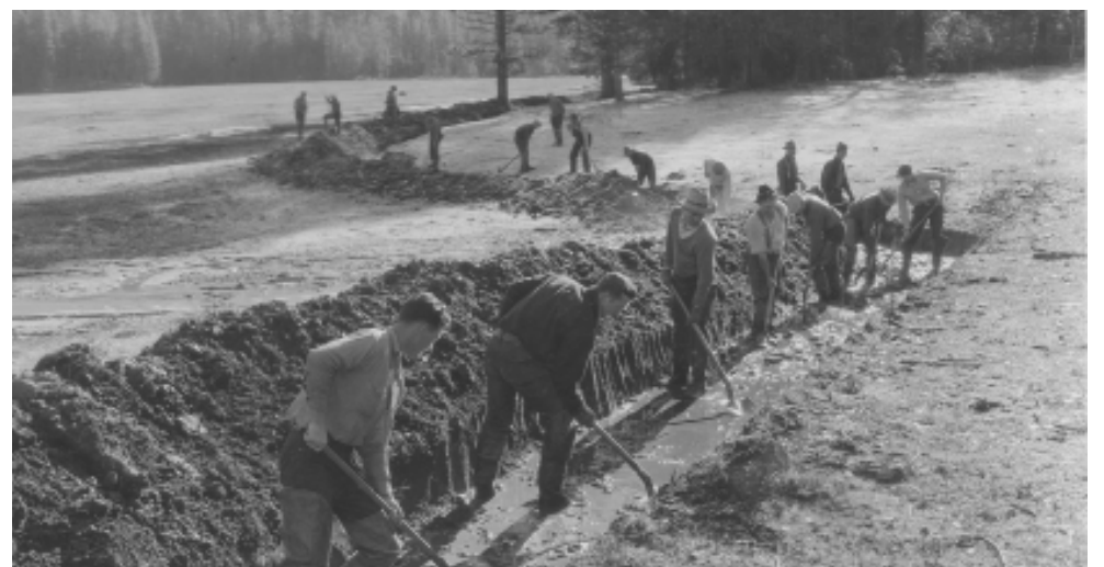
Above: CCC Workers Constructing Ditches in the Wawona Meadow, 1936, NPS Photo Top left, Gully with exposed concrete weir in Wawona Meadow, NPS Photo
