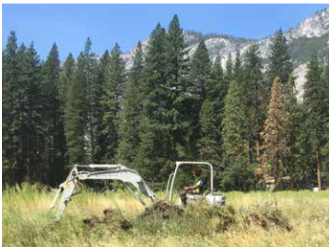
In the past, the construction of drainage ditches, trails, and roads have altered the hydrology and ecological processes of Ahwahnee Meadow. In order to improve meadow hydrology and restore meadow connectivity, native plant communities and wildlife habitat, we'll be removing conifers, drainage ditches, old road beds and social trails. NPS Photo.
