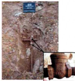
RIGHT: Crane valve on the pipe distribution system. Manufacture of this particular valve began in 1902.
