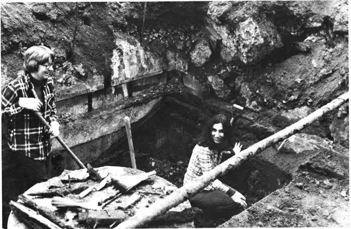
When heavy April rains caused a cave-in at Fort Point National Historic Site in San Francisco, Park Technician Cindy Orlando (right) and Secretary Trudy Allen (left) employees of the Western Regional Office joined Regional Archeologist Roger Kelly in exposing, cleaning, mapping, and back-filling the cavity that had revealed a pre-World War I military structure. However, no artifacts were found.
