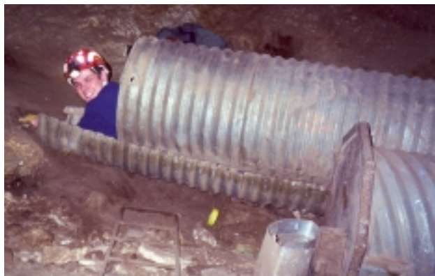
Thomas Fuller crawls through the old culvert one last time. (NPS Photo by Miho Horokoshi)
