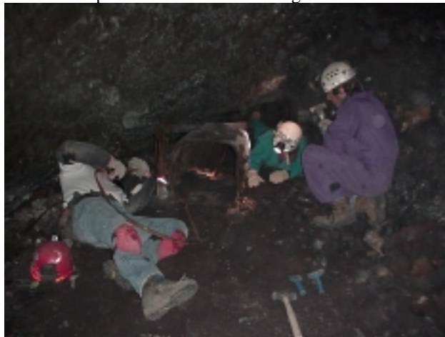
Gem State Grotto members work to remove an old gate from Arco Tunnel. (NPS Photo)
