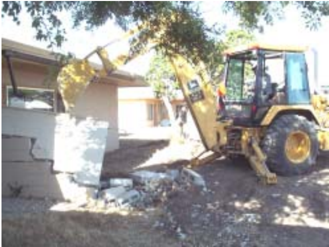
Angel Hernandez carefully demolishes a cinder-block wall associated with the Mission 66 apartments. (NPS Photo by Dale Pate)
