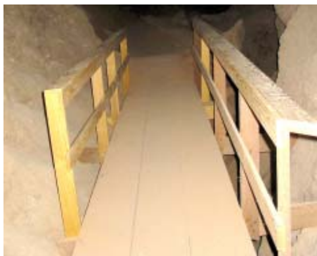
New railings have recently been installed on existing wooden structures in Left-Hand Tunnel. (NPS Photo by Tom Bemis)
