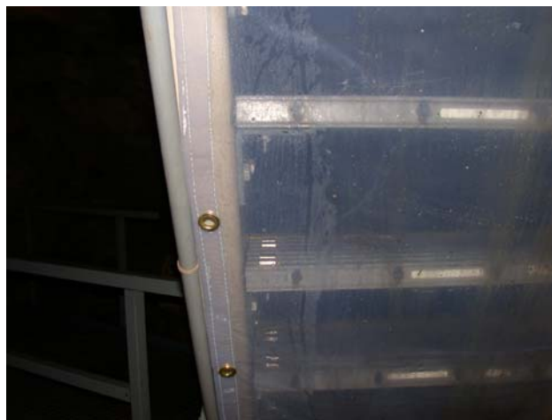
A new cave restoration supervisor position at Oregon Caves National Monument recently directed a project to install vinyl catchment tarps underneath stairs along the tour route in Oregon Caves.
