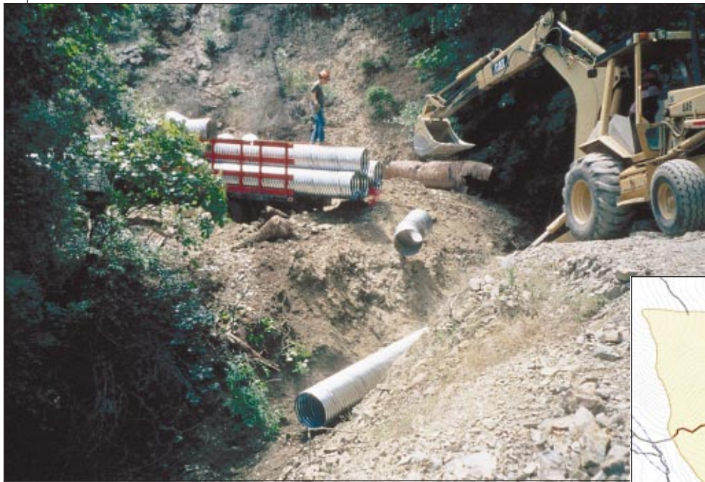
Fig. 2 (left). Heavy equipment is used to treat the drainage problems posed by the old logging roads. Here, a culvert is installed to restore natural drainage patterns and reduce erosion of the fill.
