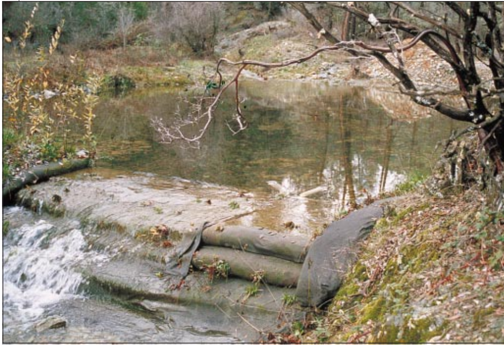
Fig. 4. A sediment pond was constructed within the lower reaches of the watershed to monitor erosion before and after restoration work. After three years, it will be removed and the stream restored to its natural course.
