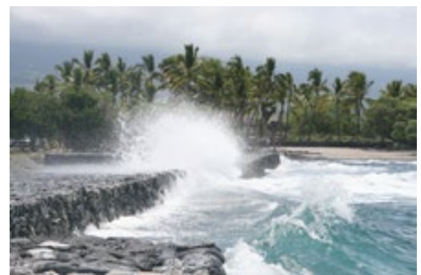
Erosion of fish pond walls at Kaloko-Honokōhau National Historical Park in Hawaii. NPS photo
