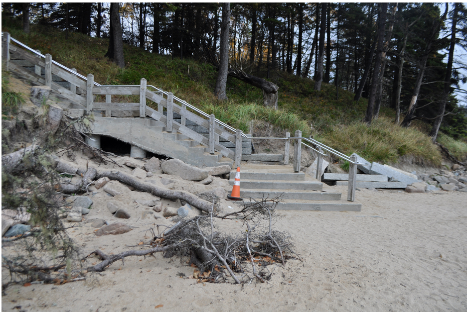
Figure 44. View looking northwest at the bottom of the staircase, showing undermined piers and retaining wall stone. A portion of the eroded bluff is visible at image left. (OCLP 2024)
