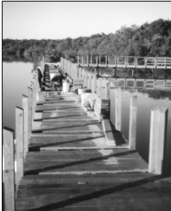
The West Lake boardwalk provides visitor access into the mangrove estuary. Rehabilitation of the boardwalk used "lumber" made from recycled materials.
