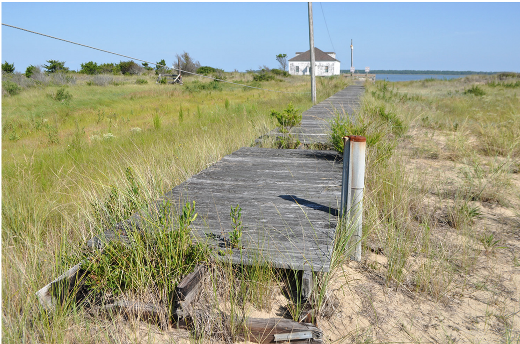
Figure 36. View looking north-northwest damaged portions of the wood walkway that connects the Station House to the facilities at Toms Cove. (OCLP 2023)
