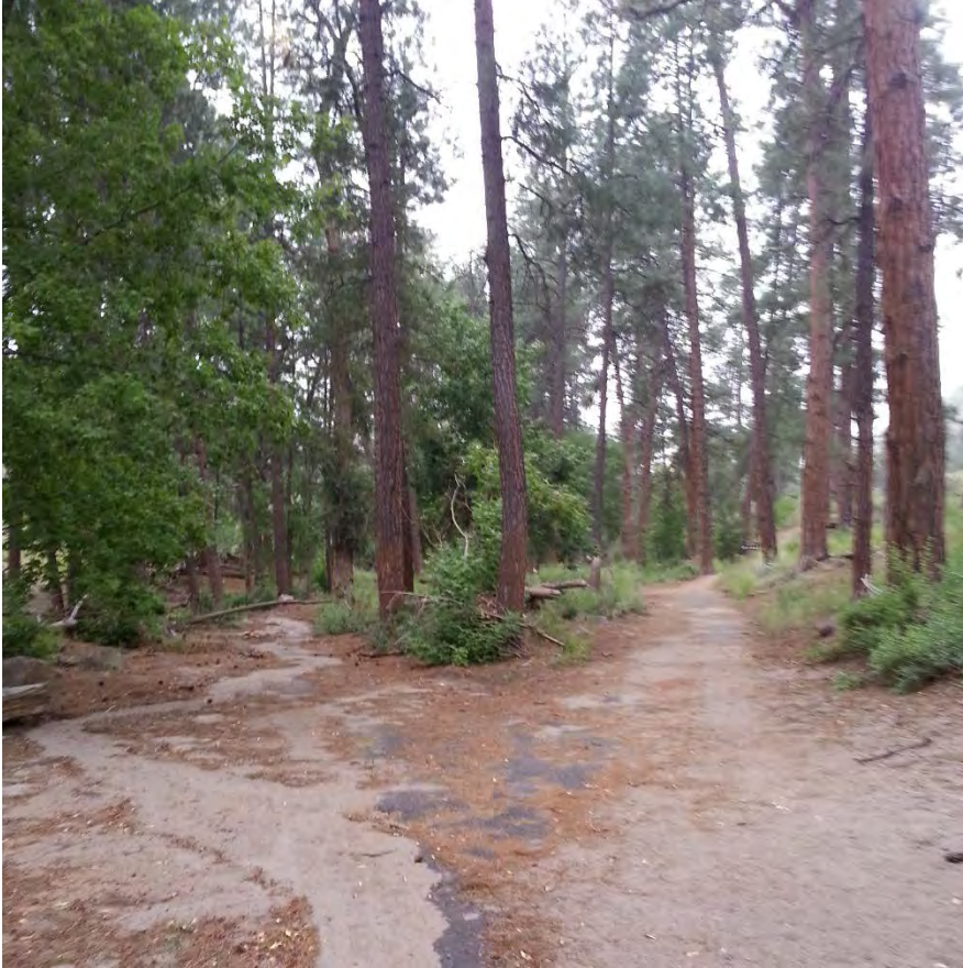
Figure 4. Damaged Section of Route 202 Needing Repair and Widening.
