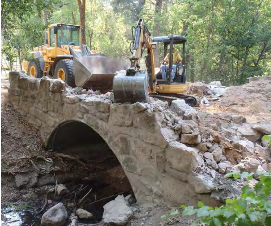
Figure 2. Removal of Old Vehicular Bridge to Reduce Flood Damage and Protect the Visitor Center.
