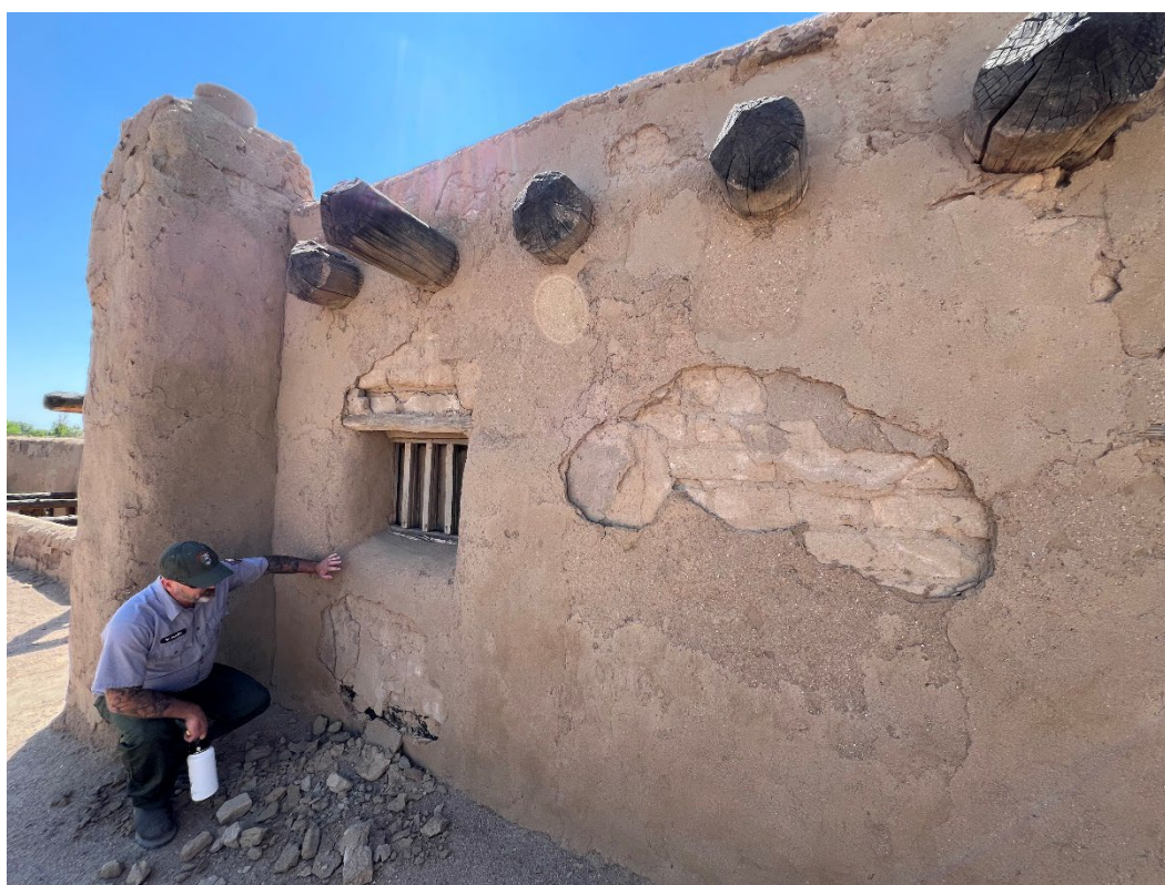
Photo Number: 5OT.1728_16 Description: Looking at the exterior wall erosion of the billiard room on the second floor. View: South
