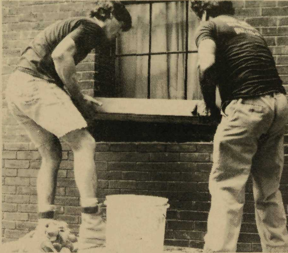
Photo #5 — Brownstone Replacement and exterior improvements on Lewis and Harriet Hayden House.
