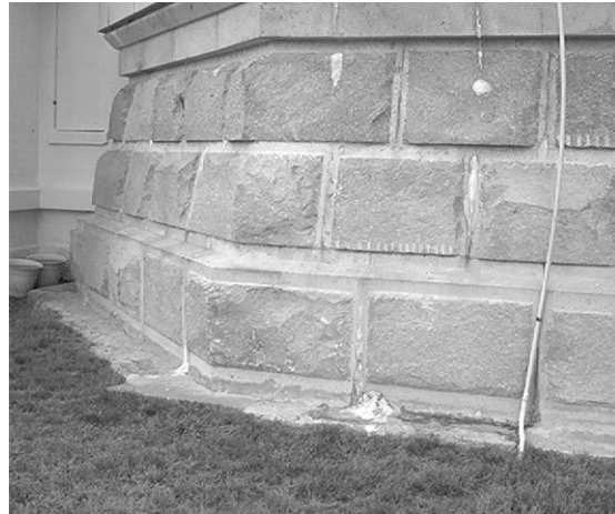
Figure 42 Conduit for lightning protection, located at tower base.
