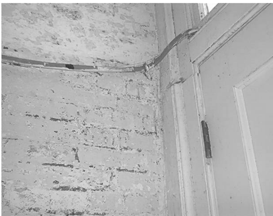
Figure 38 Detail of electrical line.
