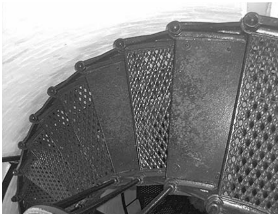
Figure 14 Existing repairs to stair treads.
