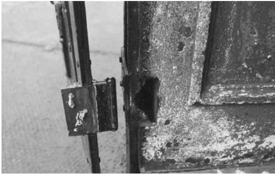
Figure 11 1989 USCOE photo showing detached hinge on door to gallery.
