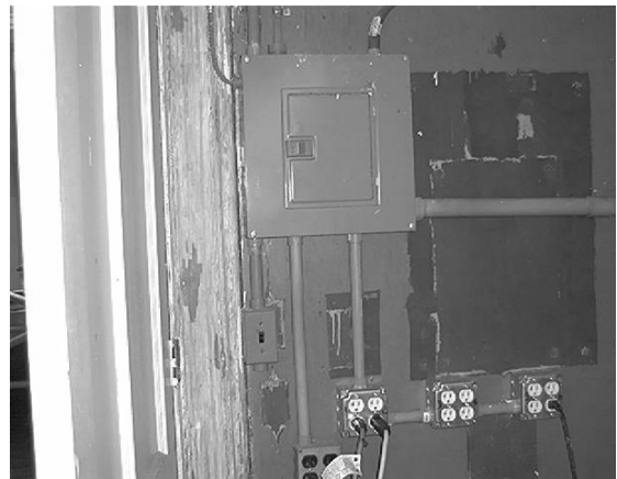
Figure 40 Detail of distribution panel.
