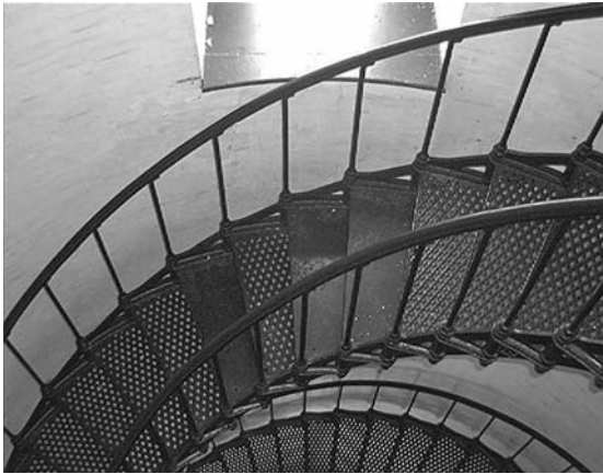
Figure 43 Detail of stair showing tread repair.
