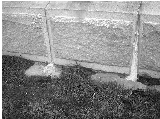
Figure 44 Detail of foundation showing mortar leaching.
