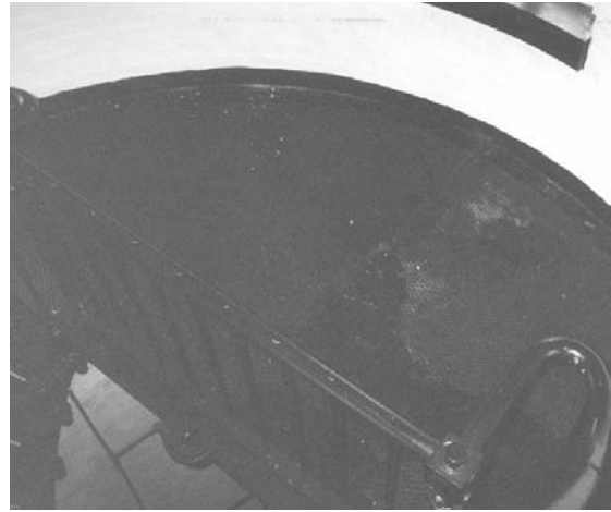
Figure 32 Detail of water collecting on landing that accesses Service Room.
