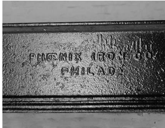
Figure 4 Landing support beams in Tower. Beams were actually installed with manufacturer's stamp upside down. Photo courtesy of Jack McCombs.
