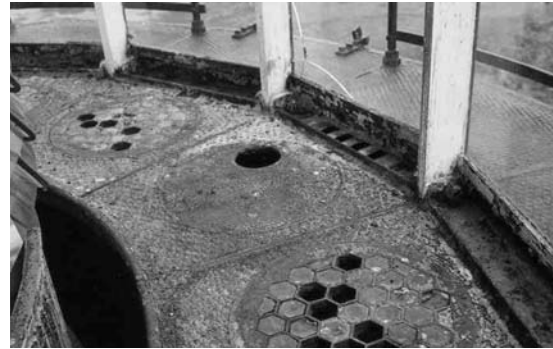
Figure 10 1989 USCOE photo showing missing lantern deck prisms.
