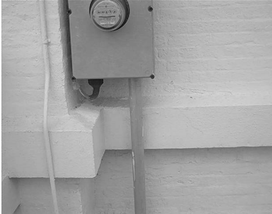
Figure 36 Detail of utility meter.
