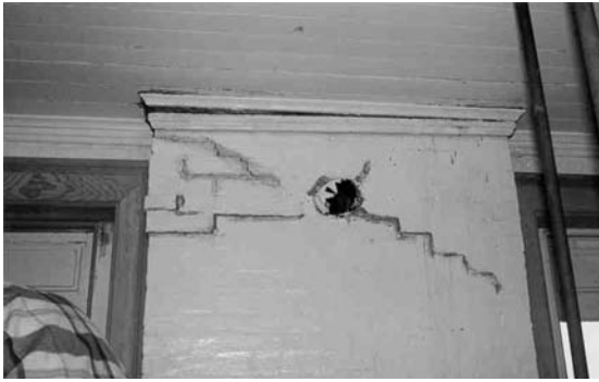
Figure 8 1989 USCOE photo showing cracked masonry in Oil Room interior chimney.
