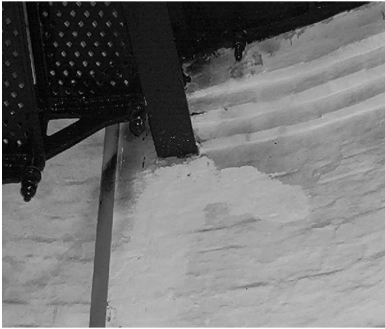
Figure 31 Detail of masonry repair located above landing support beam.
