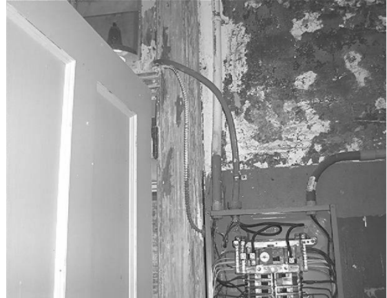
Figure 39 Detail of electrical wiring access to distribution panel.
