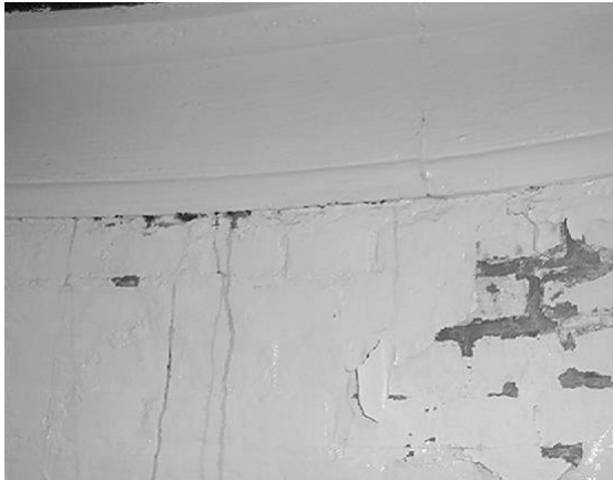
Figure 33 Detail of peeling paint in Watch Room.
