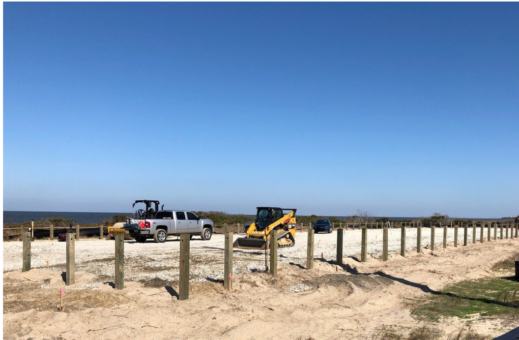
The Kite Point parking area project is progressing well. It is anticipated to open in the coming weeks.
