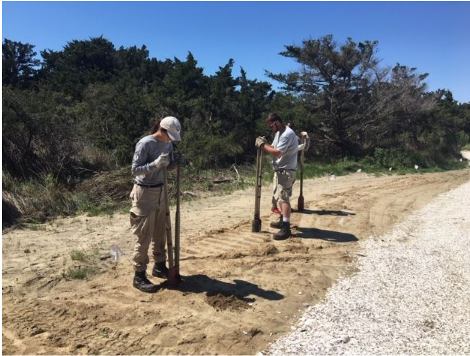
AmeriCorps NCCC team preparing to install bollards along Devil Shoals Road on Ocracoke Island.
