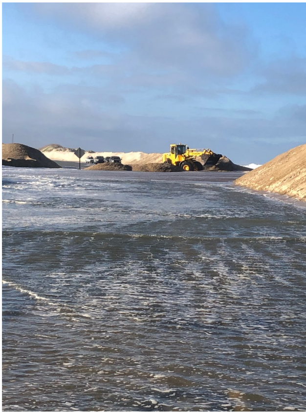
NC Department of Transportation crews worked hard to fortify the dunes north of Rodanthe last week. Dune breaches, including a 60-to-80 foot breach, caused multiple NC-12 closures.
