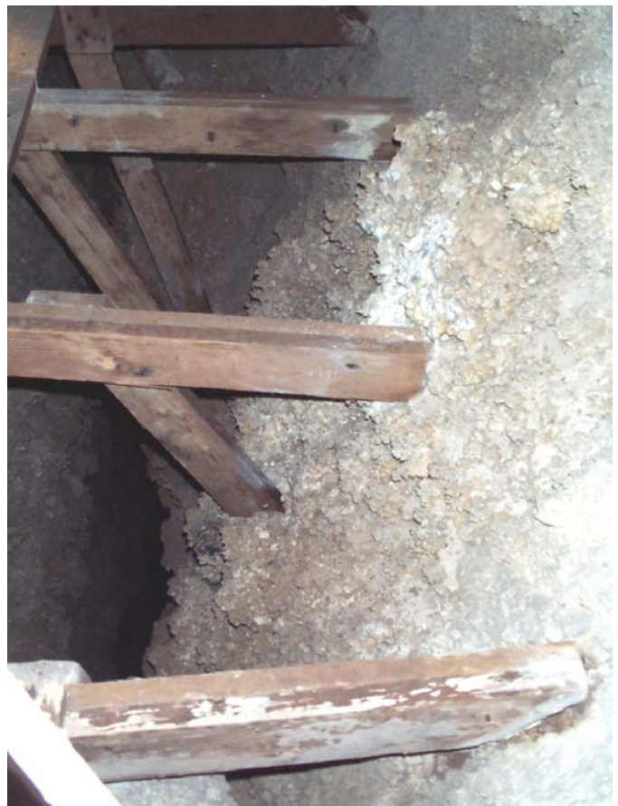
The bridge is held in place by large 4" x 6" and secondary 2" x 6" braces jammed into the walls of the pit.
