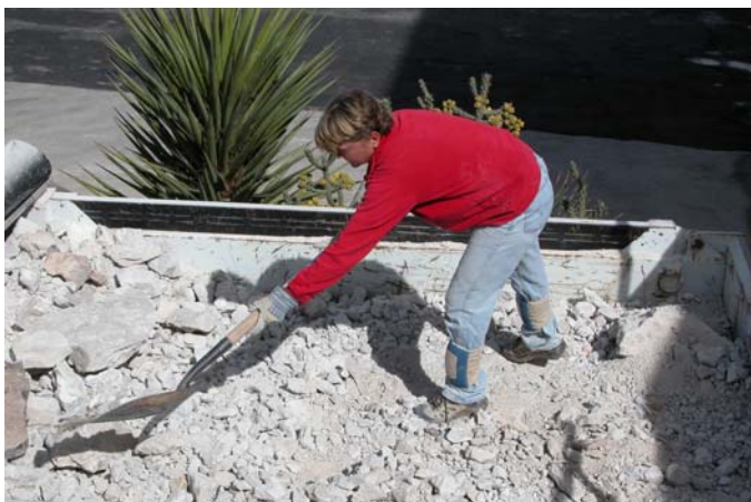
Rebecca Lee packs rubble into the back of the dump truck. (NPS Photo by Dale Pate)
