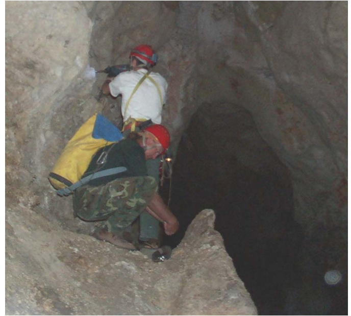
Stan Allison and Bob Kobza placing a stainless steel expansion bolt for the traverse line.
