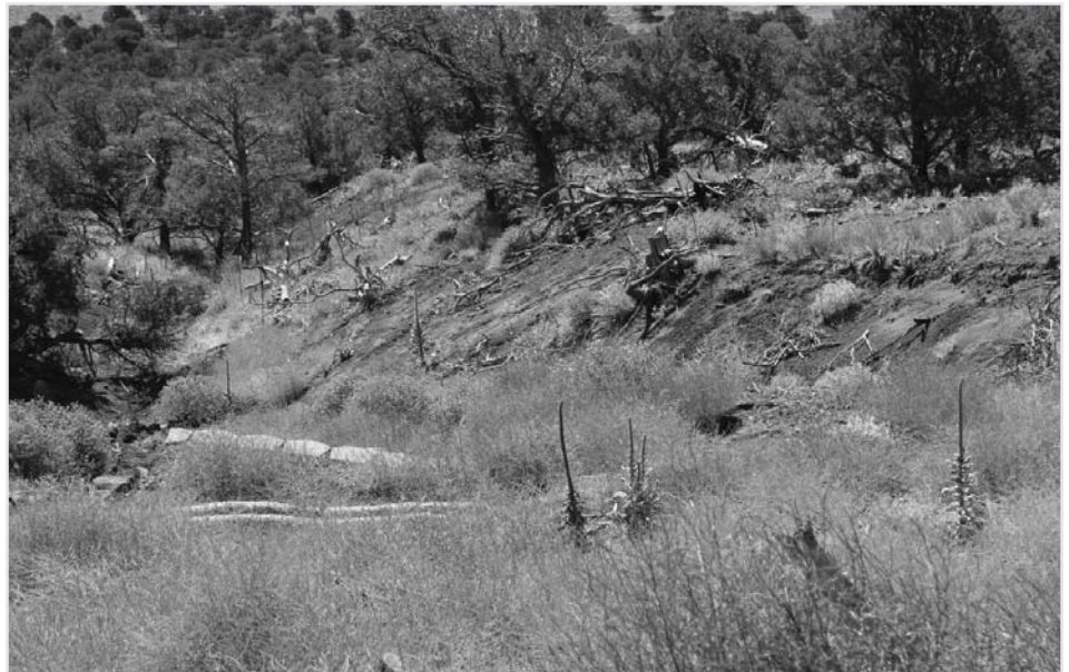
Culvert 14, one of several inadequate culverts, has experienced significant erosion due to heavy rainfall undermining the road to the volcano rim. Notice the exposed cinder.
