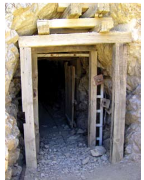
Mine adits and shafts are potential death traps and should not be entered.
