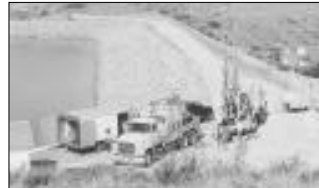
The Great Plains Regional drill crew performed investigative drilling. Photo by Lovell Parish
