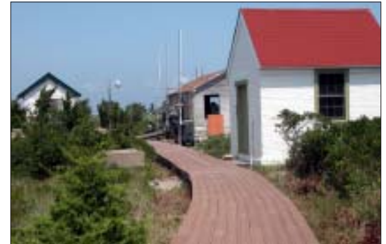
Plastic lumber sheathing was installed on some of the boardwalk at the lighthouse tract.
