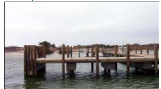
The Barrett Beach ferry dock was designed and built to withstand severe wave action at its location, one of the broadest parts of the Great South Bay. This is also the narrowest part of Fire Island.
