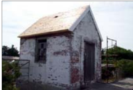
The old boathouse (top), the historic oil house (above: "before"; right: "after"), and other outbuildings were painted and some were reroofed this year.
