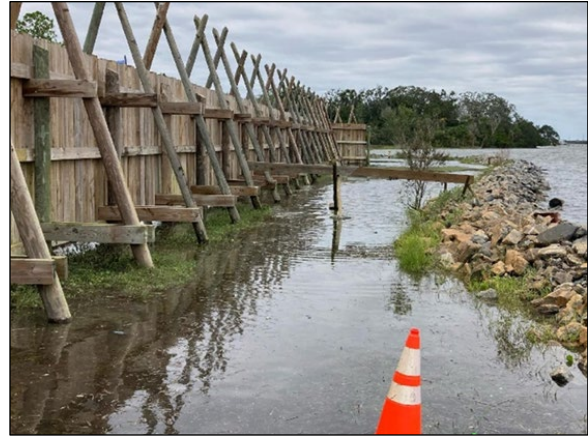
Figure 3. Flooded Walkway Between St. Johns River and Fort Exhibit
