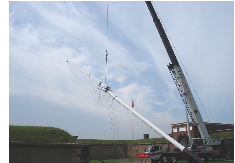
The new flagpole is hoisted into the Fort, the temporary flagpole is seen in the background.
