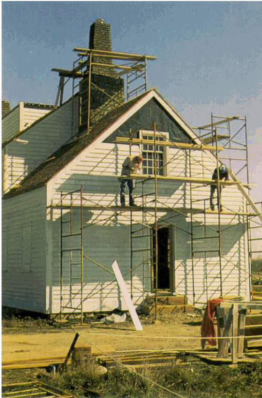
Bourgeois House under construction in 1987. (Fort Union Trading Post, A Pictorial History, MWRO. Photo by Richard Cronenberger, NPS.)
