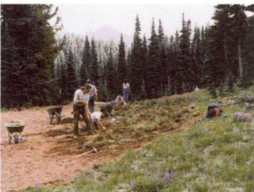
NPS personnel work to revegetate a disturbed area of Mount Rainier National Park, Washington.
