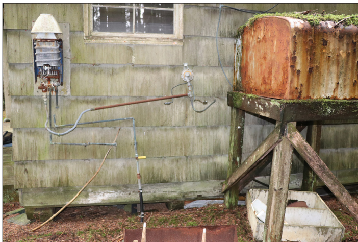
Figure 8.22: The North Elevation of the Lagoon Island includes the mechanical systems including an oil fired hot water heater, 100-gallon fuel tank supported by an untreated timber frame and regulators with copper tubing for appliances at the interior. All of the equipment has exceeded its useful life and will require replacement.
