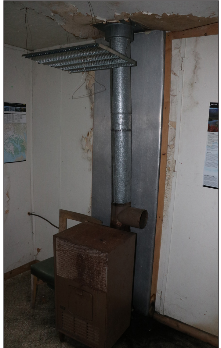
Figure 8.23: The primary heat source for the Lagoon Island Cabin was an oil-fired heater located in Room Two which no longer functions. Oil leaks have damaged and stained the floor and water leaks from the vertical exhaust vent has damaged the ceiling and walls.
