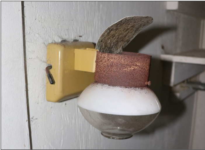
Figure 8.21: The interior was most recently illuminated by wall mounted propane lights. Rehabilitation efforts may include an electrical system powered by intermittent use of a generator or a power source from the mainland. The system is yet to be determined.
