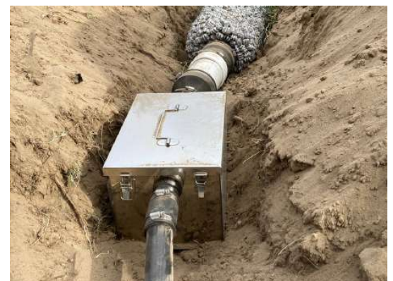
Silver Drainfield - Rocky Flats Campground, WA
