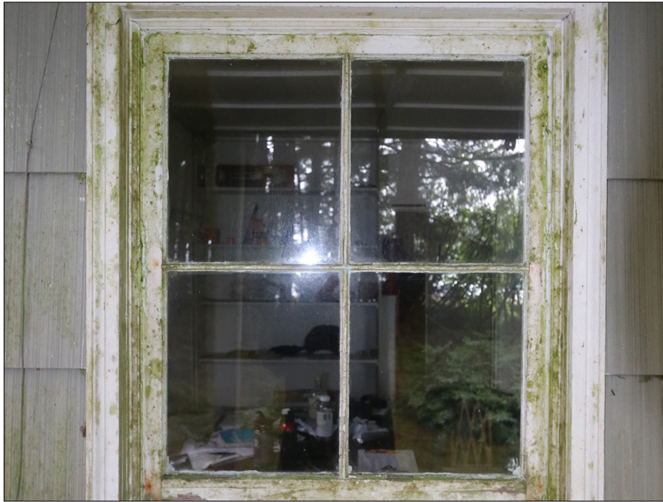
Figure 8.12: Typical fixed, wood sash 4-lite window located on the east elevation to the north of the primary door. The windows remain in sound condition despite the moss growth.
