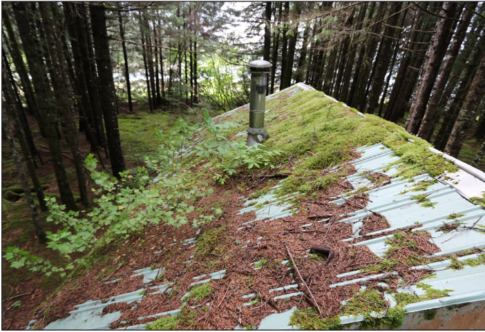
Figure 8.6: The roof was covered with duff, moss and vegetation during the 2018 site visit. Park staff cleared the debris shortly after the site visit. The aluminum roof is programmed for replacement in 2025.
