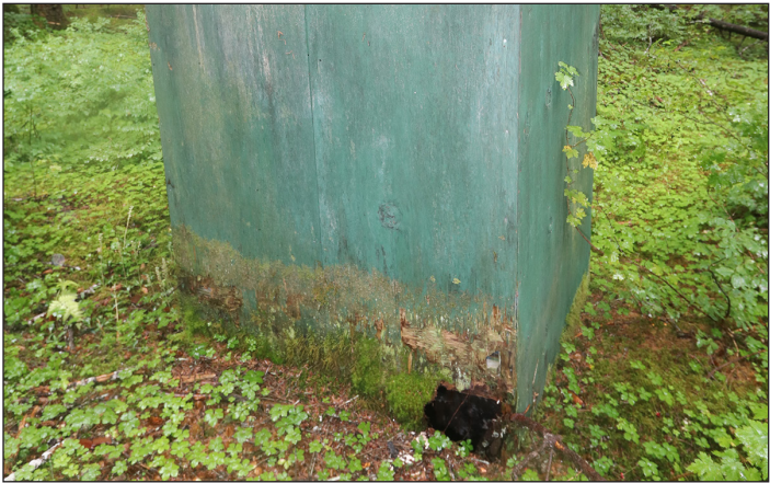
Figure 8.26: The North elevation has deteriorated at the corner. A new outhouse will be required for the cabin site.
