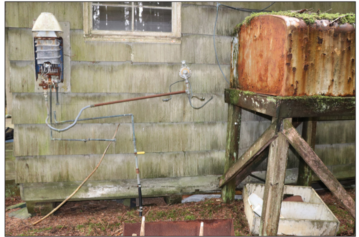
Figure 5.33: The south elevation of the cabin includes the mechanical systems including an oil fired hot water heater, 100-gallon fuel tank supported by an untreated timber frame and regulators with copper tubing for appliances at the interior. All the equipment has exceeded its useful life and will require replacement.
