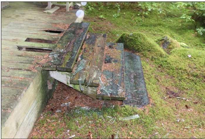
Figure 8.15: View of the deteriorated stairs at the cabin's primary entrance.
