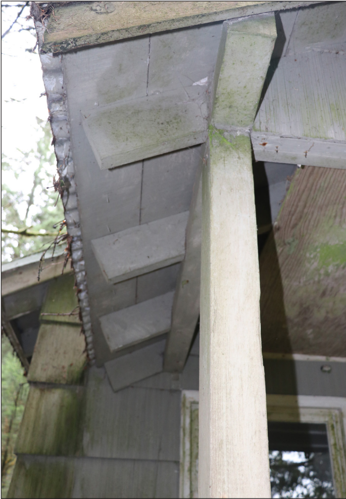
Figure 8.10: View of the porch roof north eave assembly which remains in sound condition despite some moss growth which can be mitigated with simple cleaning and repainting.
