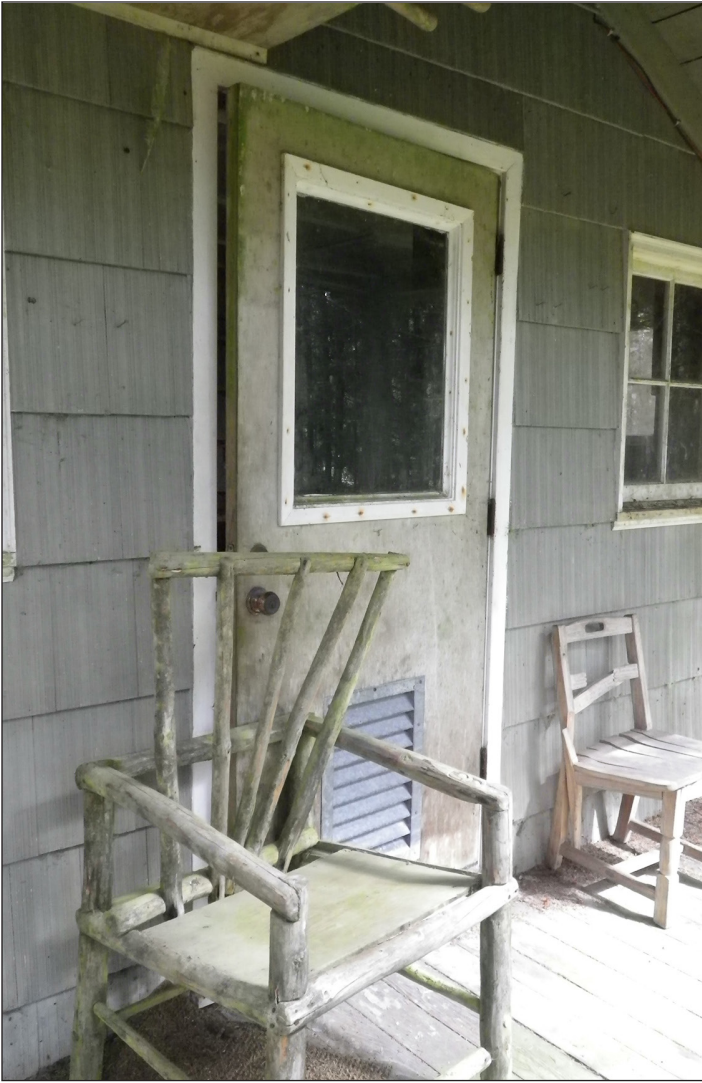
Figure 5.10: The door serving the primary entry to the cabin on the south elevation was a half-lite, solid core door. The door was vandalized in 2018. Following the vandalism incident, the park installed plywood until the final preservation treatment is realized. NPS Photo, 2013.
