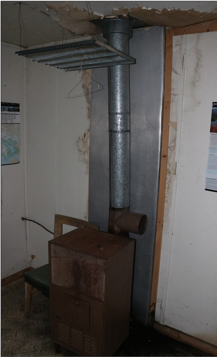
Figure 5.32: The primary heat source for the Lagoon Island Cabin was an oil-fired heater located in Room 2 which no longer functions. Oil leaks have damaged and stained the floor and water leaks from the vertical exhaust pipe has damaged the ceiling and walls.
