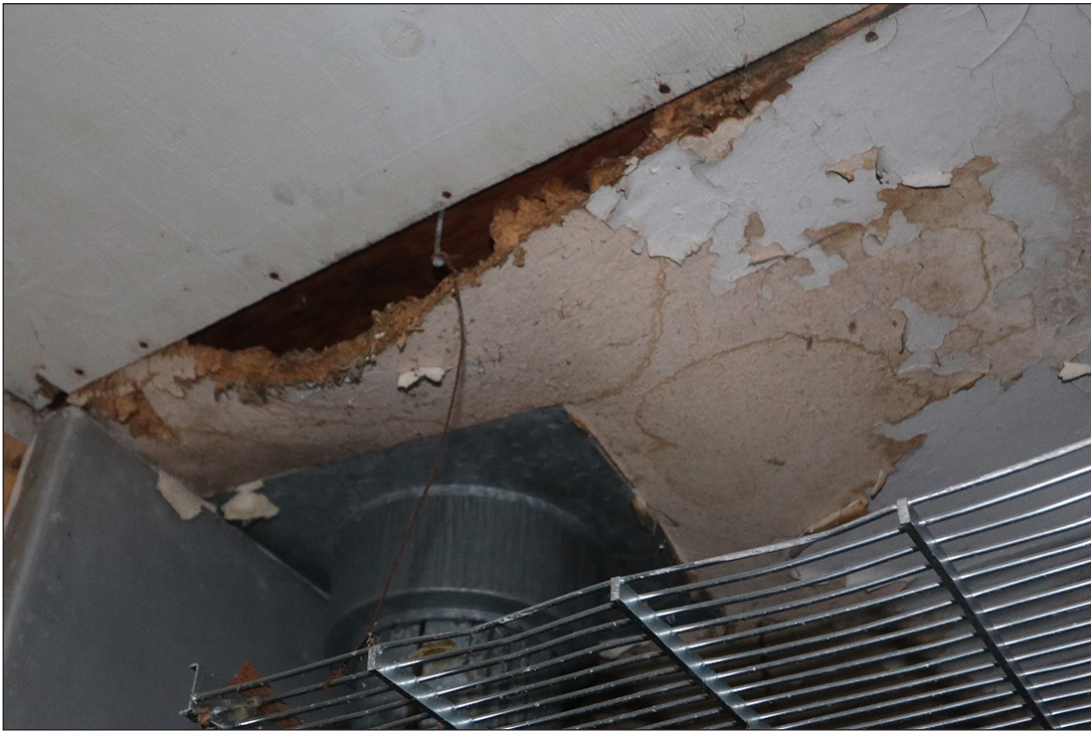
Figure 8.5: The ceiling around the gas stove has deteriorated beyond repair. The attic appeared dry during the 2018 inspection.
