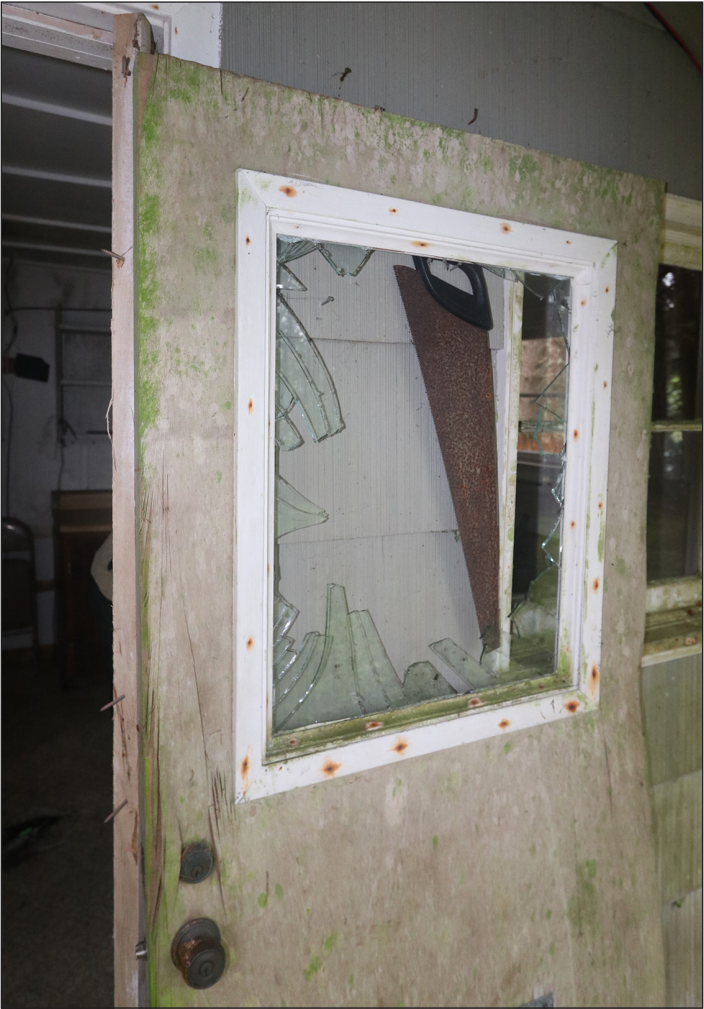
Figure 8.11: The door serving the primary entry to the cabin on the south elevation was vandalized in 2018. The door was severely damaged and is no longer serviceable. Following the 2018 site visit for this HSR, park facilities staff installed plywood over this entrance as a stabilization measure. Plywood remains in place and a period appropriate door will be specified when the project proceeds.
