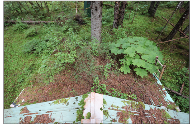
Figure 8.9: View to the east from atop the primary roof. The shed roof addition is completely covered with duff and actively supports vegetation.
