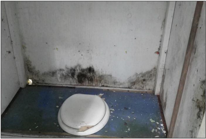
Figure 8.25: Interior view of the existing outhouse with mold growth at the interior.
