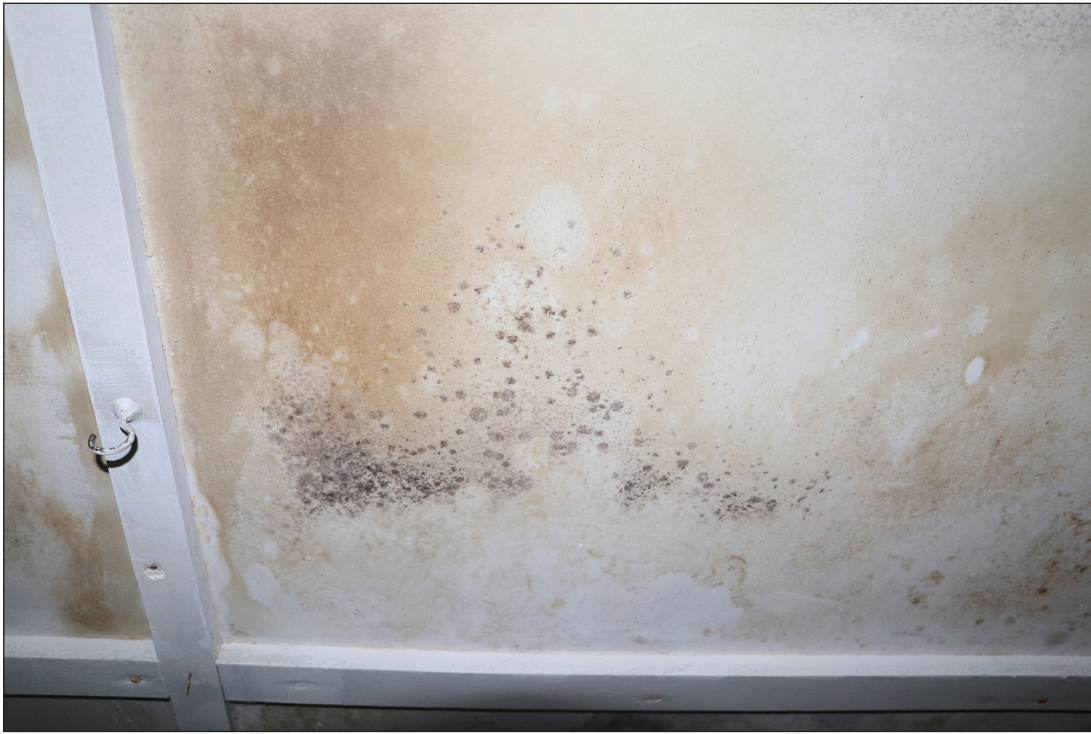
Figure 8.4: The ceiling and a few locations on the walls are stained and have mold growth.
