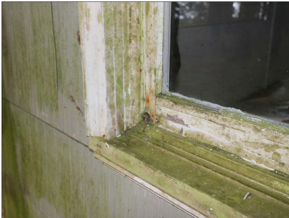
Figure 8.13: Detail view of the window sill pictured above illustrating the moss growth on the wood sill and sash.
