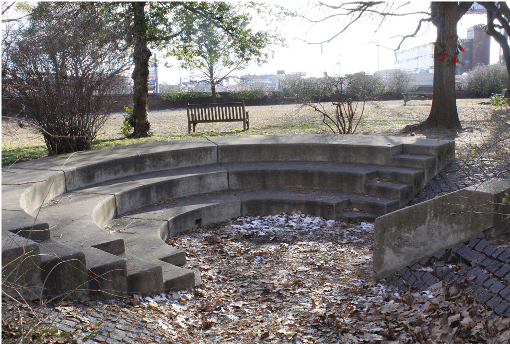
Figure 48. Amphitheater, view looking south, built by the NPS in late 1970s. Slatted seat boards, light sconces, and a memorial plaque on the plinth (image right) are missing, and leaf litter likely clogs the floor drain. A bench is visible in the background. (CLR 2022: 152)
