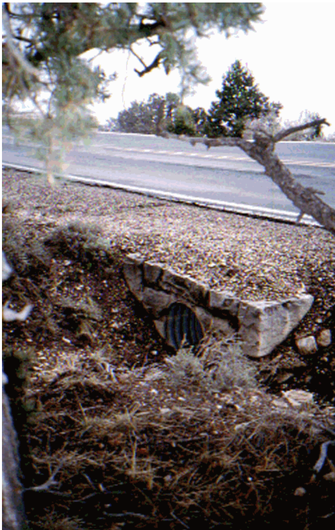
Culvert allowing drainage under West Rim Drive. (Photo by J. Galbraith, 2003)
