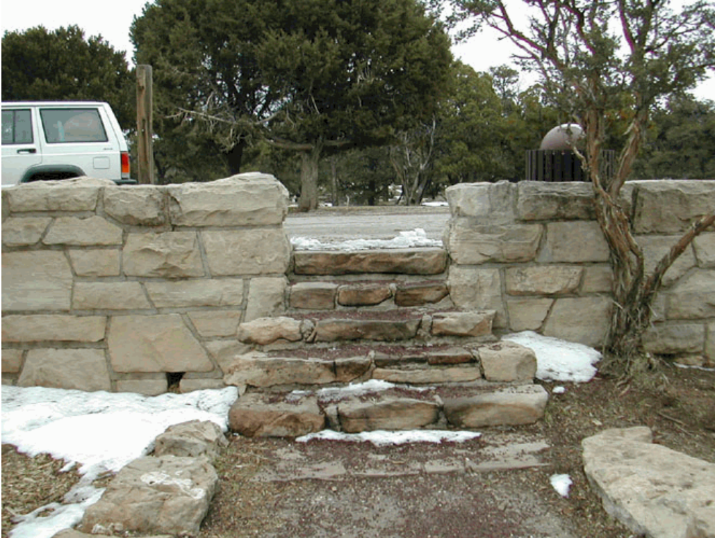
Masonry steps and walls found at the major overlooks along West Rim Drive. (Photo by J. Galbraith, 2003)
