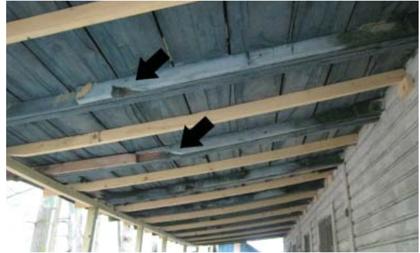
Figure 15. Roof rafters of front porch. Added rafters terminate at a bird-mouth cut.
