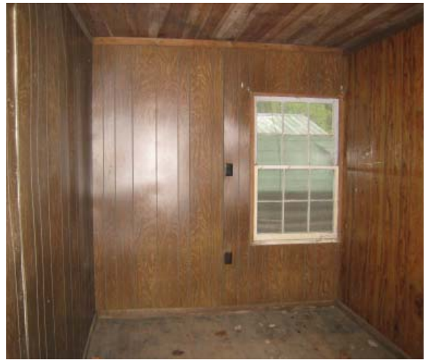
Figure 38 , Northeast oblique of Room 101 with modern veneered wall panels. Note that window casing has been removed to install wall panels.
