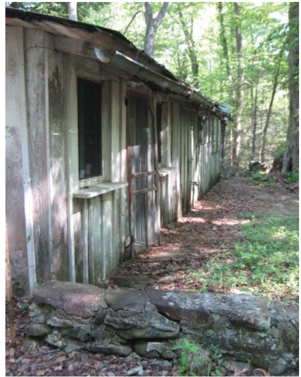
Figure 78 , Failed roof gutters, unpainted and deteriorated wood elements and loose stone site features.
