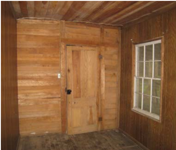
Figure 40 , Southwest oblique of Room 101. Early wall on left with exposed studs and beaded boards. Wall on right covered with modern veneer paneling.
