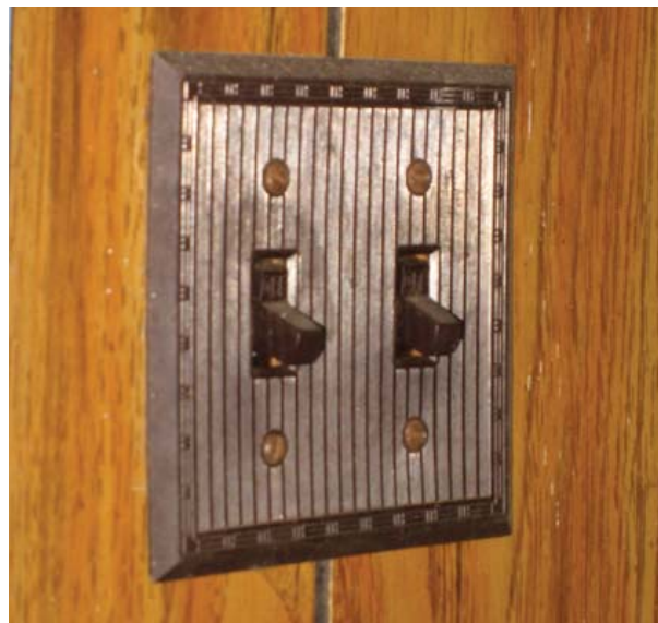
Figure 18, Typical mid-twentieth century molded plastic switch and outlet cover.
