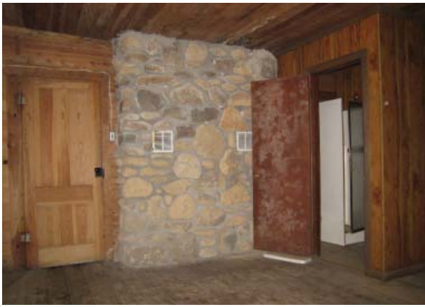
Figure 51 , Northeast oblique view of Room 104, master bedroom, with master bathroom, Room 105, to right, chimney stack in the center and original four-panel door at left connecting to the living room, Room 103.
