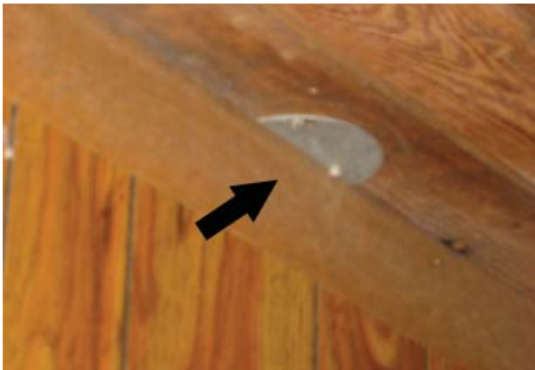
Figure 45, Metal cover for earlier ceiling fixture at wall between Room 101 and Room 102.
