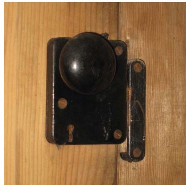
Figure 30 , Original steel rim lock with mineral doorknob at doors of main block.
