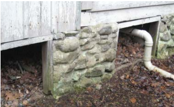
Figure 14. Stone foundation pier at north elevation spans between Northeast Bathroom on left and main block on right.
