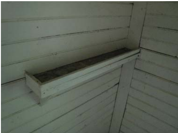
Figure 68, Wall shelf at foot of bath tub.
