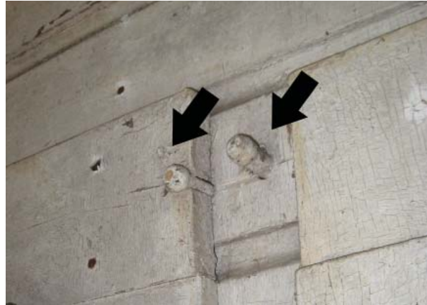
Figure 17, Two porcelain tubes in west wall are remnants of early knob-and-tube wiring.
