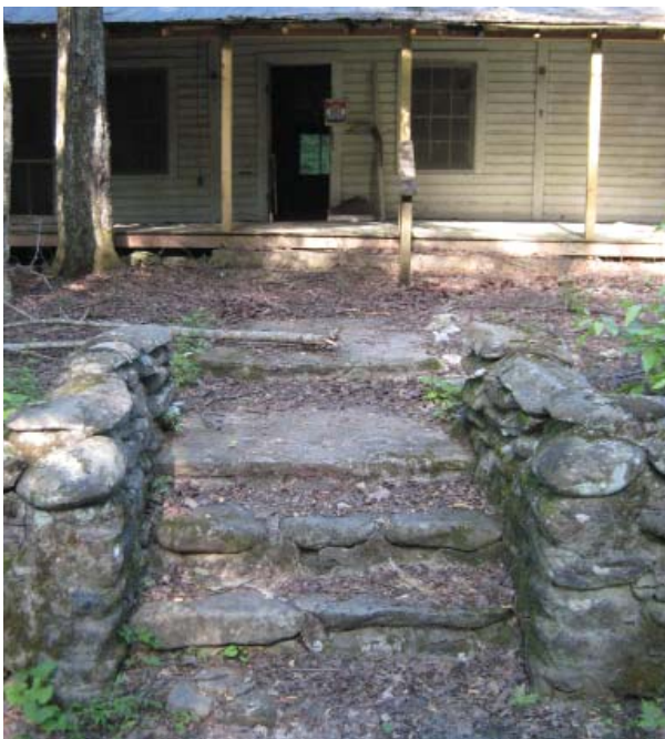
Figure 3, Front entrance steps leading to walkway skewed to center doorway of Addicks Cabin.
