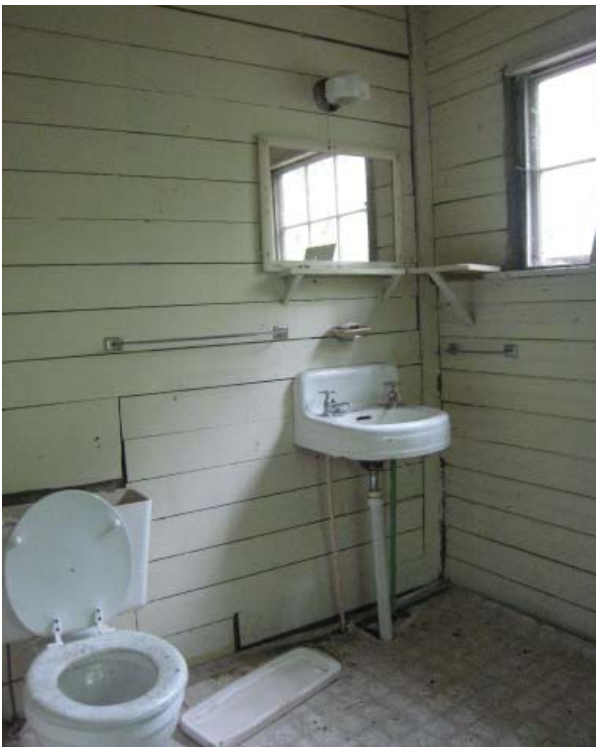
Figure 64, Northwest oblique of Room 108, northeast bathroom with early plumbing and lighting fixtures.
