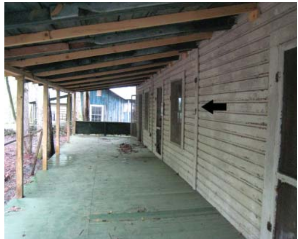
Figure 9 , Front (west) elevation of main block of Addicks Cabin with plank boards covering seams in German siding.
