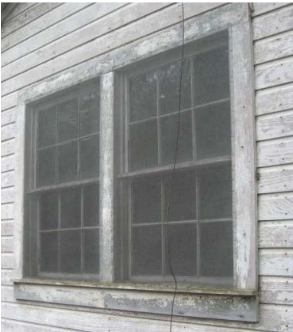
Figure 25 , Original double-hung windows paired on the north elevation of the main block.
