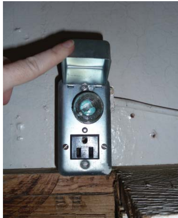
Figure 82. A three-prong outlet with fuse on north wall of Room 105.
