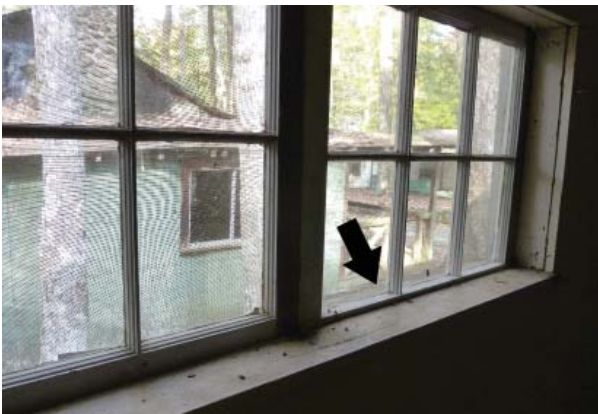
Figure 53. Recently repaired window of the north elevation that is lacking the Type A profile.
