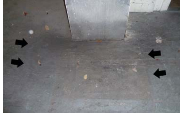
Figure 39. Discoloration of flooring indicating the location of a wood-burning stove, Room 104.
