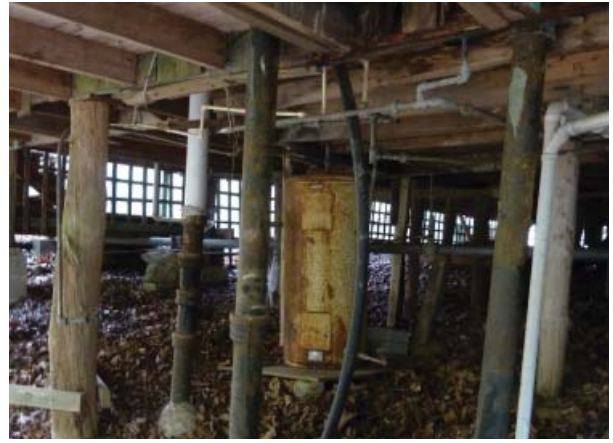
Figure 42. Inoperable electric hot water heater in the crawl space.
