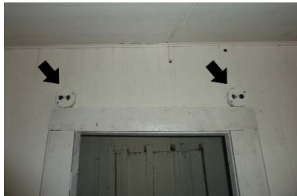
Figure 69. Duplex outlets mounted above the doorway on the west elevation, Room 102.
