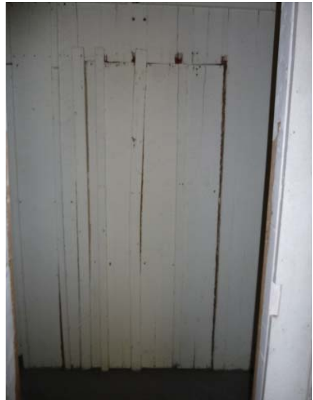
Figure 98. West wall of Room 109a with seams for an opening to allow for installation of the tub in Room 108.
