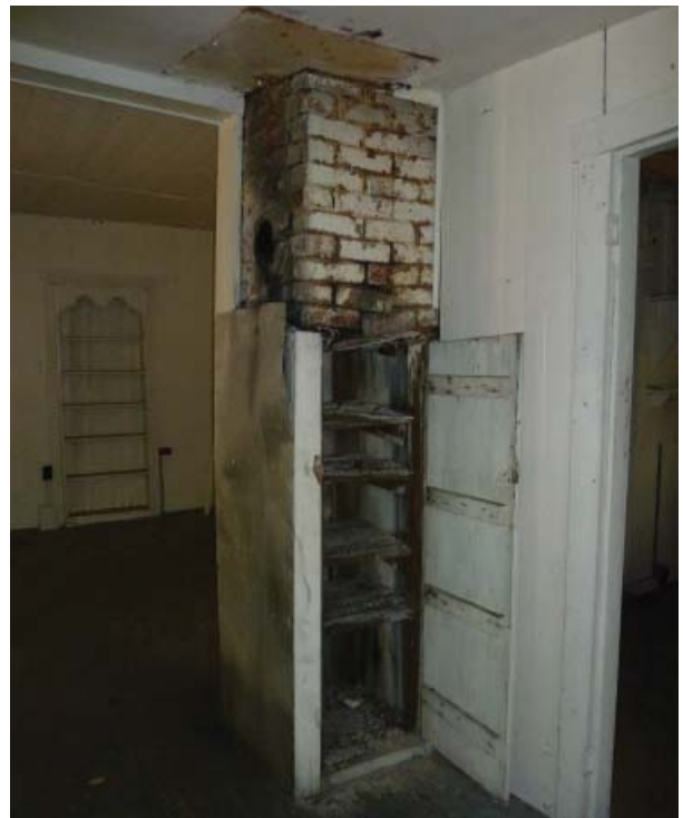
Figure 76. Chimney supported by built-in wooden cabinet in the southwest corner of Room 104.
