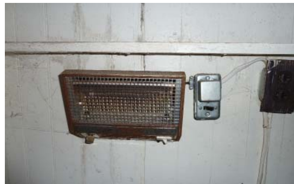
Figure 40. Electric heater used in the bathrooms.
