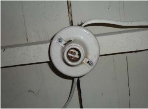
Figure 41. Typical ceiling-mounted ceramic lamp holder used in most rooms of the cabin.
