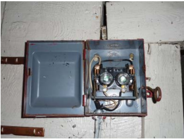
Figure 83. Fuse box on the south wall of Room 105.
