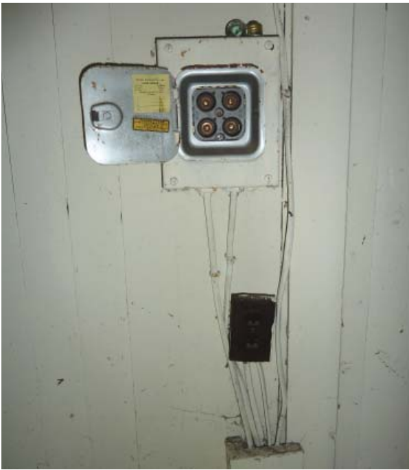
Figure 64. Fuse box and duplex outlet on the south wall.
