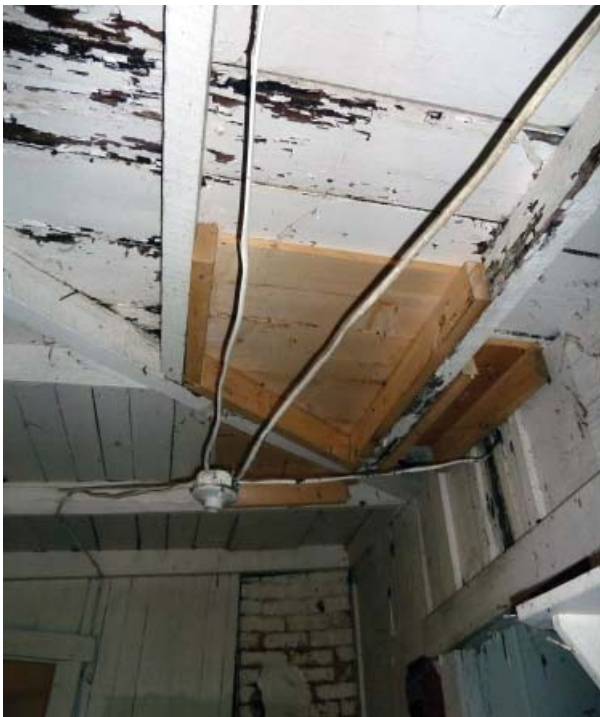
Figure 81. Exposed roof rafters and various areas of ceiling repair in Room 105.
