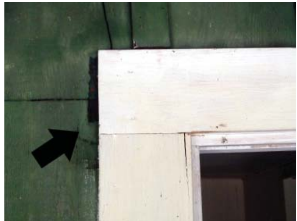
Figure 48. Exterior door casing of front door with paint remnants indicating size of earlier trim board.
