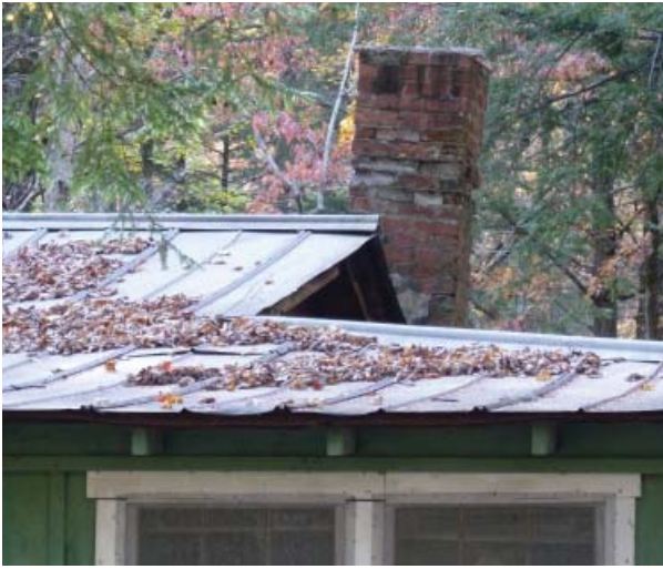
Figure 46. Brick chimney that is leaning to the north.
