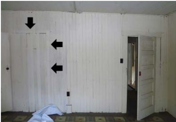
Figure 61. Rooms 101a & 101b looking north. Infilled door patch (left) mirrors door opening (right).
