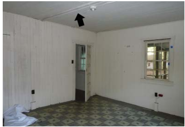
Figure 59. Southeast Bedroom (Rooms 101a & 101b) looking northeast. Only the header of the north-south dividing wall remains.
