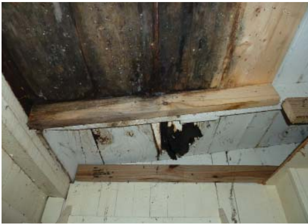
Figure 95. Exposed roof rafters and decking with various repairs in Room 108.
