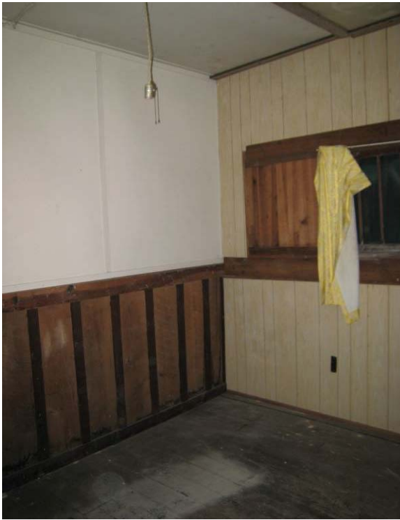
Figure B- 9. Early board-and-batten wainscot on the left wall with later gypsum board-and-battens above. The right wall has been covered with 1/8" laminated hardboard paneling. The ceiling is likewise covered with later gypsum board-and-battens.
