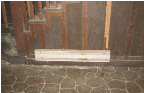
Figure C- 70. Mid-century baseboard heater.
