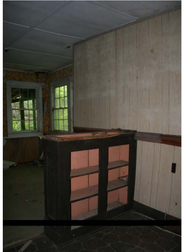
Figure C- 21. Cabinet at northwest corner of Room 101.
