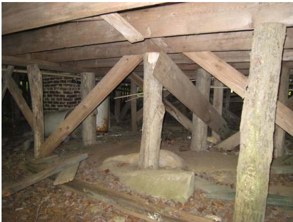
Figure C- 2. A variety of support posts and bracing in the crawl space.
