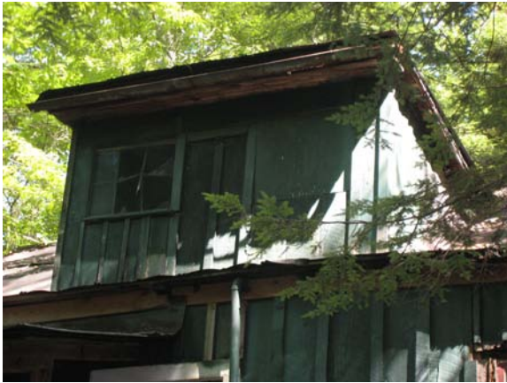
Figure B- 6. West elevation dormer showing wood panel covering previous window opening.
