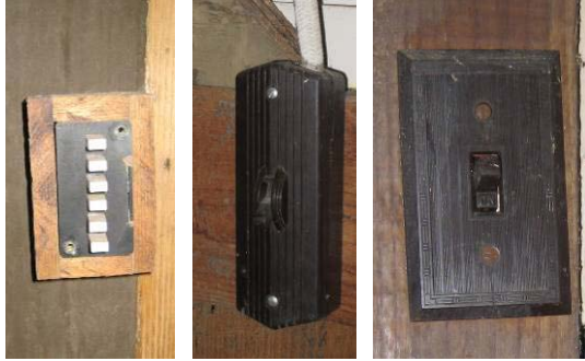
Figure B- 11. Variety of light switches found in the Cabin.
