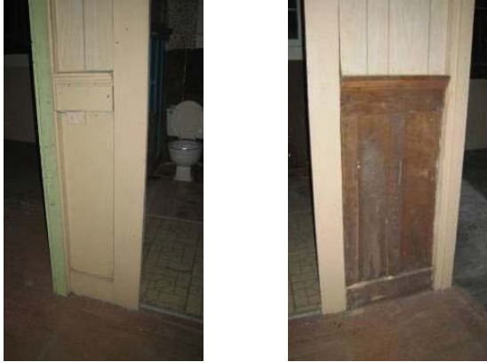
Figure C- 36. South wall of Room 106, showing different wainscot on either side of Room 105 doorway.
