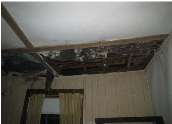
Figure C- 31. Water damage to ceiling in Room 104.
