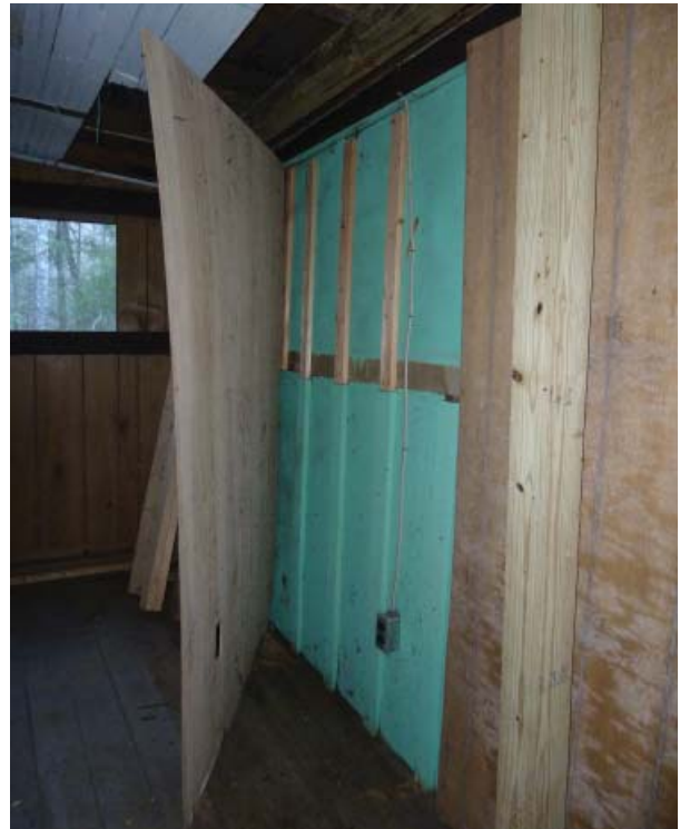
Figure 82. Paneling delaminating from wall of Northwest Bedroom (Room 105).
