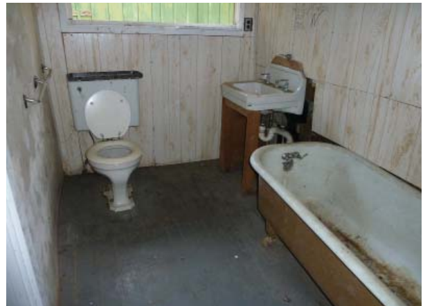
Figure 53. Plumbing fixtures of the Bathroom (Room 109).
