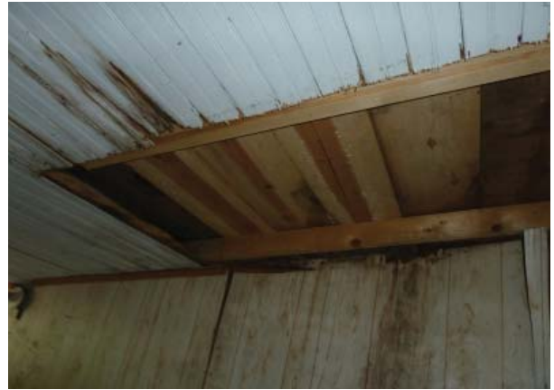
Figure 98. Patch in northwest corner of the ceiling.
