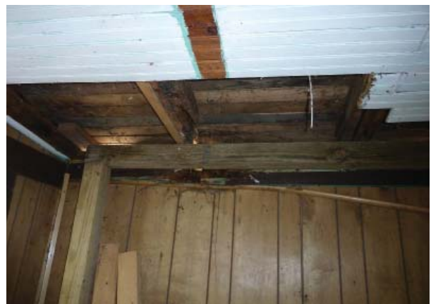
Figure 83. Poor condition of ceiling in Northwest Bedroom (Room 105).
