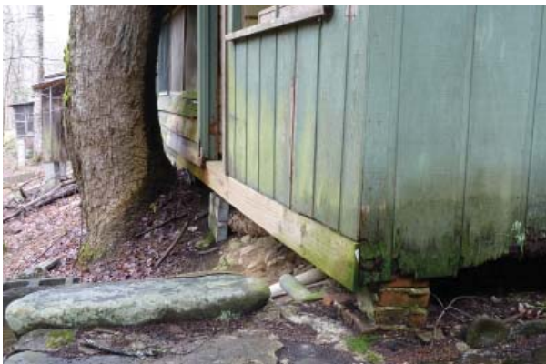
Figure 55. Southwest corner of cabin, location of collapsed deck.
