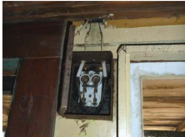
Figure 50. Early fuse box with ceramic tubes in Living Room (Room 102).
