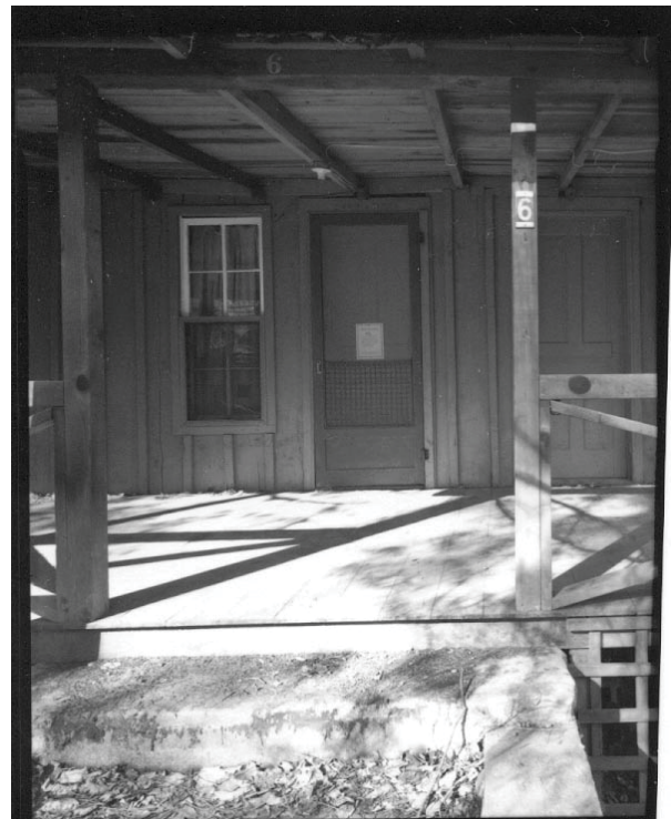
Figure 35. Gutter above entrance bay of front porch. Note the house number 6 above the entrance, and another on the north post of that bay. (HABS-250-G-11)
