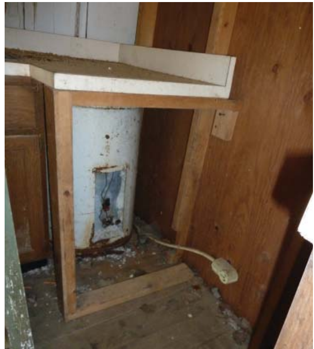
Figure 52. Inoperable hot water heater in the Kitchen (Room 108).
