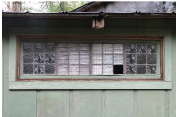
Figure 65. 36-light window on the south elevation, now missing.
