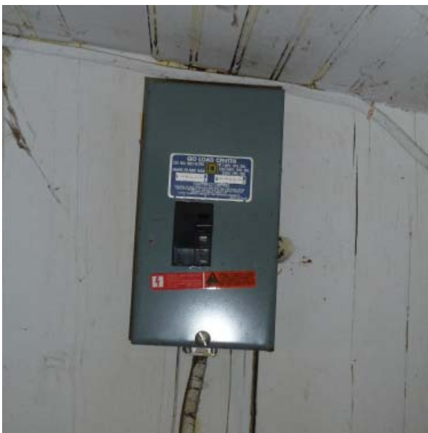
Figure 95. Electrical panel on the east wall of the Kitchen (Room 108).
