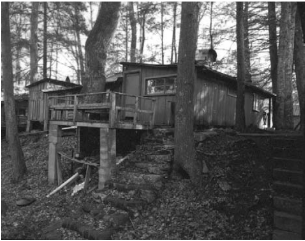
Figure 25. Raised deck at kitchen door seen in 2001, when the tall CMU piers are near collapse. (HABS-250-G-8)
