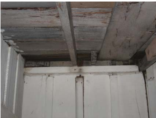
Figure 7 , The consistency of the two rafters and roof sheathing north of Room 104 appear to indicate an earlier room or porch.
