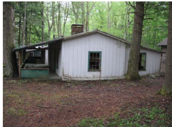
Figure 5, South elevation. The shed-roofed southeast wing (Room 104) is at right; offset about 2 feet from the main block.
