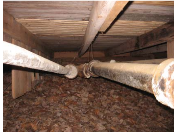
Figure 54, Galvanized (left) and cast-iron (right) waste lines leading from the bathroom, view toward north. Note the replacement flooring in Room 103, beyond, due to water damage. The band joist for the addition is attached to the original Servants' Quarters at left.
