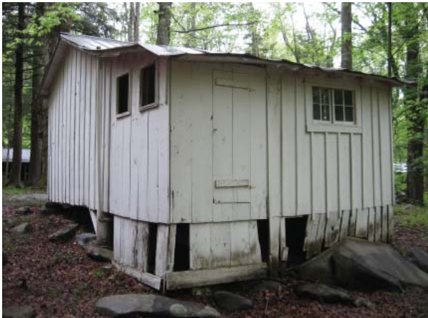
Figure 47 , Southeast oblique. The northeast corner (right) bears directly on the rock outcropping. Note the use of locust post piers and wood board underpinning.
