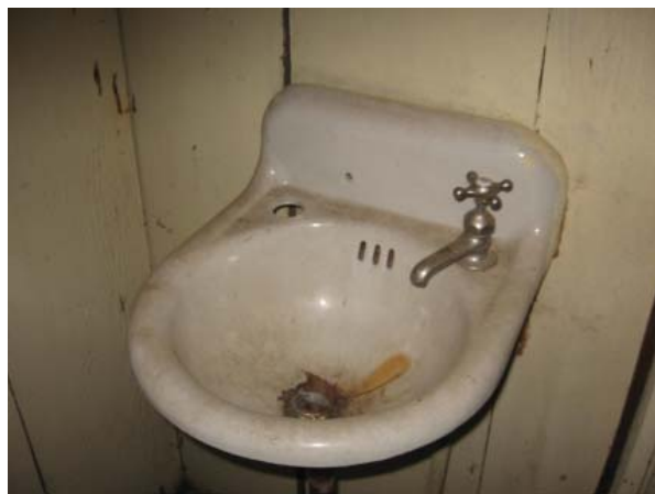
Figure 44, Cast-iron lavatory at Room 104.
