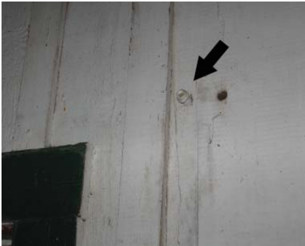
Figure 12, Porcelain tube in west wall is a remnant of early knob-and-tube wiring.
