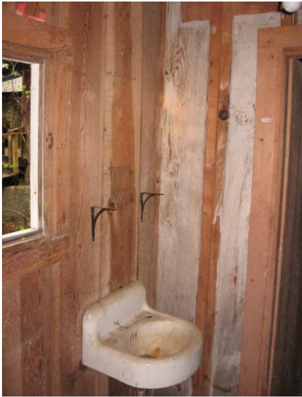
Figure 62 , Bathroom, 102, view toward west. Note that battens have been removed on the original exterior east wall of the Servants' Quarters, as seen by the paint lines.
