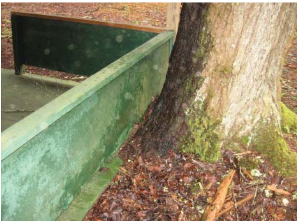
Figure 45 , South end of Front Porch where hemlock has grown into floor structure.
