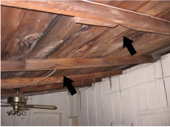
Figure 6 , The rafters in Room 103 extend from the east wall of the main block (right). The bird's-mouth cuts in the rafters indicate the presence of an earlier beam or wall.
