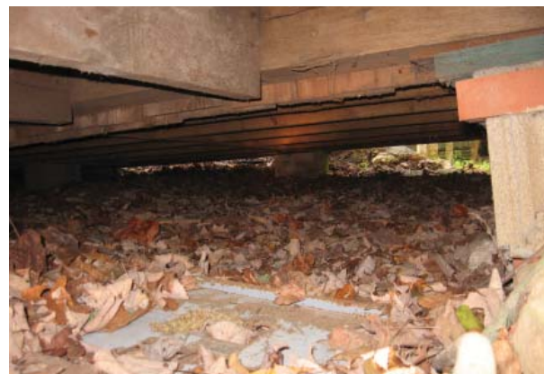
Figure 11, Floor framing under North Parlor, looking west toward front porch. Note that floor joists toe-nailed into 8" by 8" hewn sill. Vertical board wall structure can be seen on far side of sill.
