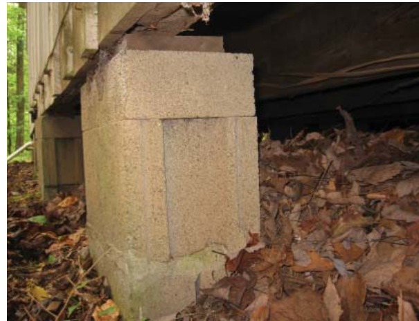
Figure 10, Typical concrete block foundation pier, north wall. Some of the piers are capped with solid 4" blocks.
