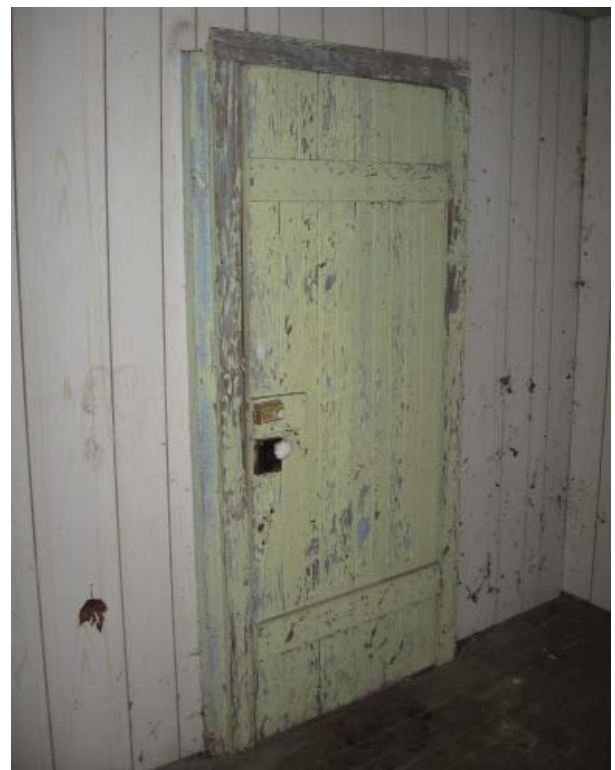
Figure 60, Door to front porch, showing projection of frame into Room 101.
