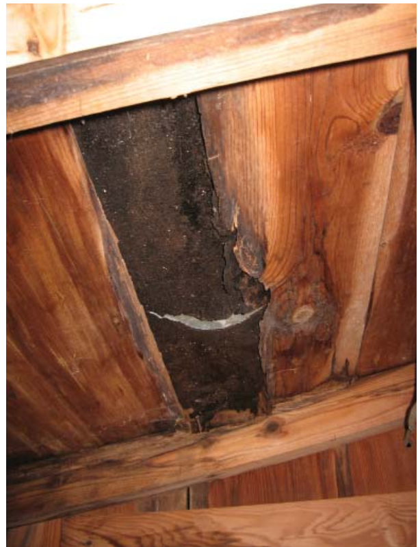
Figure 68 , Damage to roof sheathing over partition between Room 102 and Room 103.
