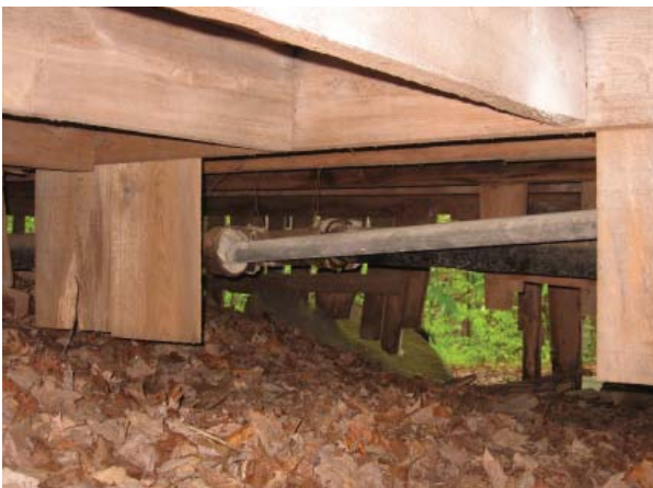
Figure 50 , Crawl space below Room 101, view toward east. Wood slat underpinning and framing for rear addition can be seen in background. The vertical boards in the foreground appear to have been used for shimming out the band joist of the addition from the wall of the original Servants' Quarters. See also Figure 54.
