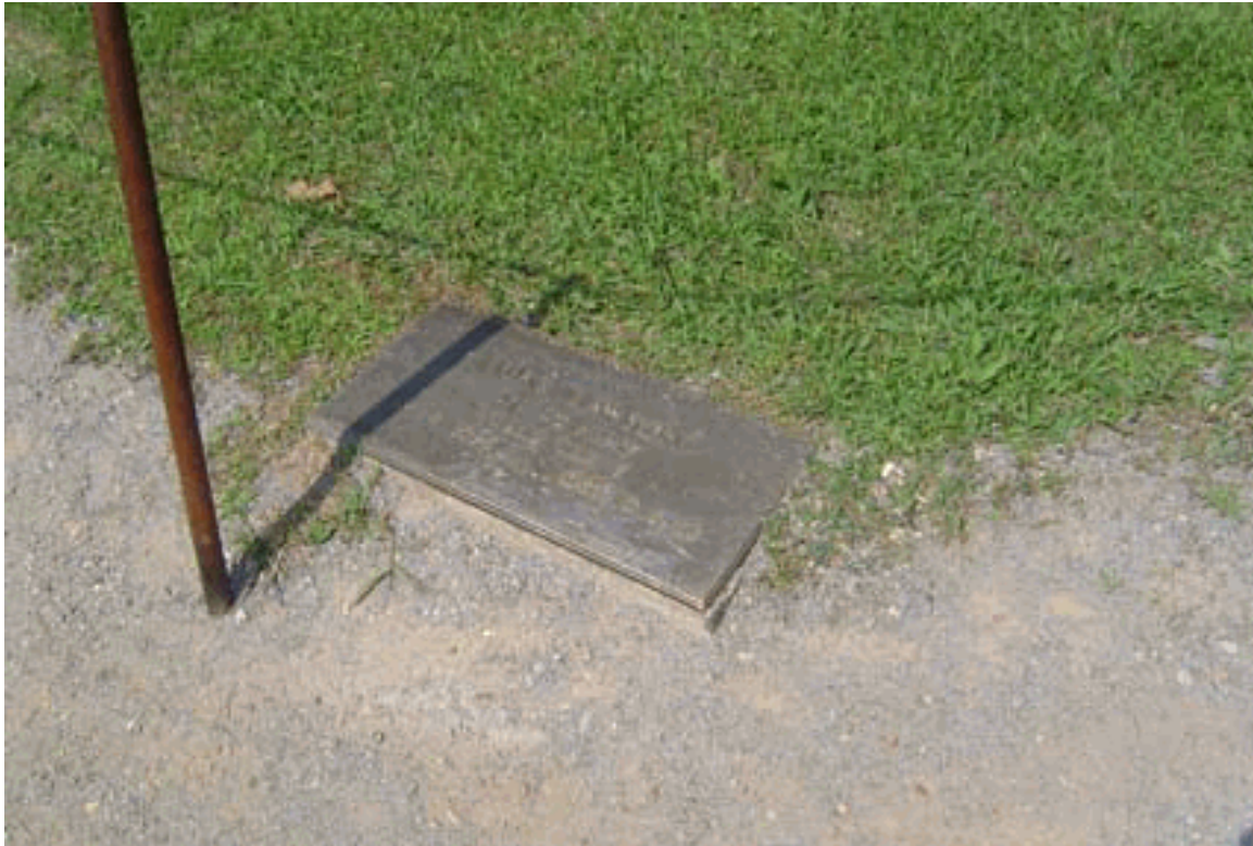
Pea gravel pathway with fencing. Note erosion around headstone (2006).
