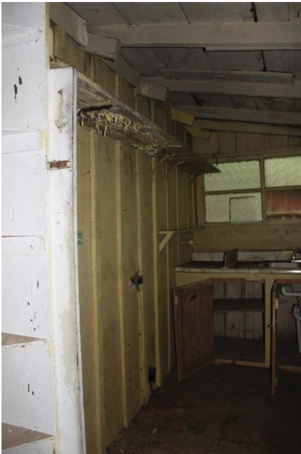
Figure 48: Room 108, rear board-and-batten wall of main core and gabled roof rafter ends.
