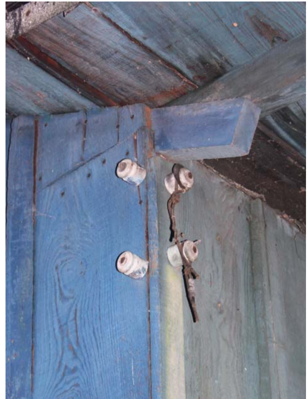
Figure 16: Remnants of ceramic knob-and-tube wiring system.
