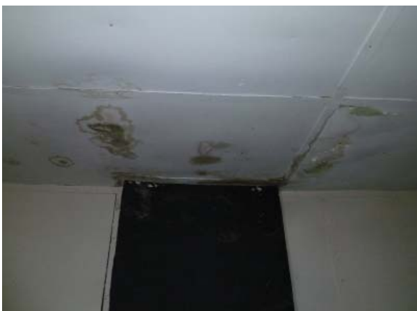
Figure 71. Severe deterioration of ceiling at chimney.
