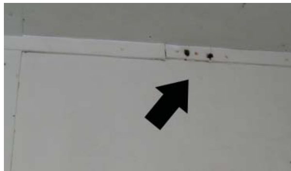
Figure 41. Holes near ceiling for early knob-and-tube wiring.
