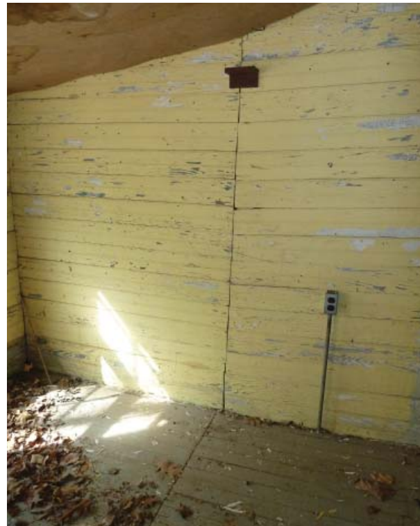
Figure 87. Vertical seam in north wall.
