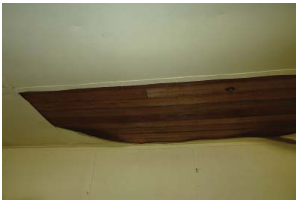
Figure 76. Damaged finish material in southwest corner of ceiling.
