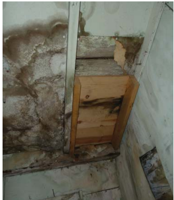
Figure 79. Severe deterioration in northeast corner of the ceiling.
