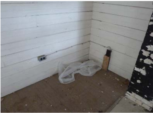
Figure 67. Electrical box and duplex outlet in the northwest corner of the room.
