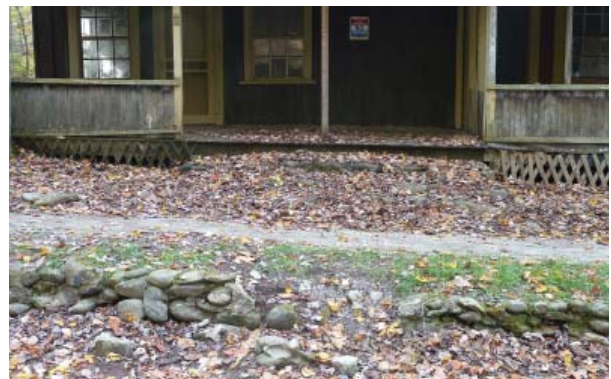
Figure 28. Partial collapse of retaining wall in front of Smith Cabin.
