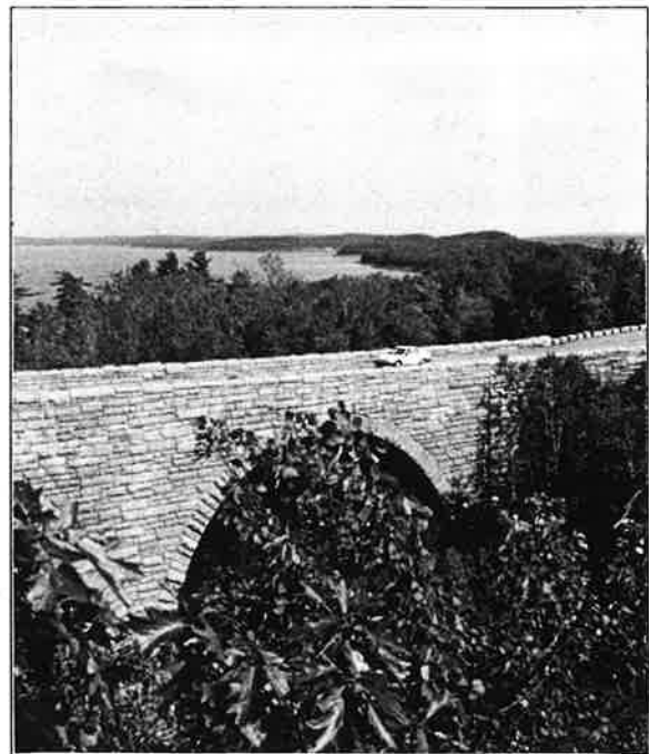
Paradise Hill Road Bridge, on the Historic Motor Road System, Acadia National Park.
