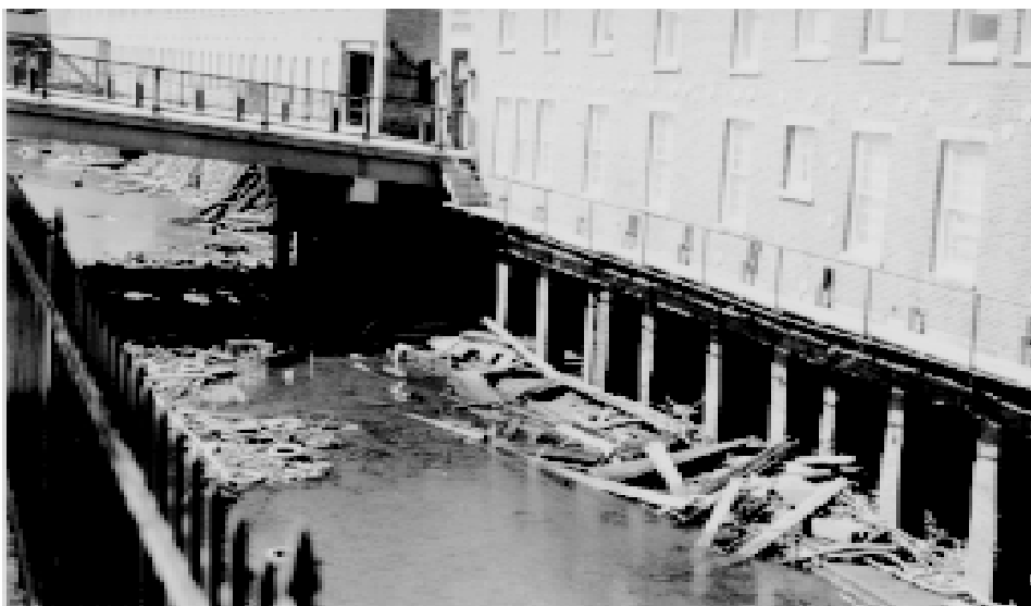
Draindown reveals trash on bottom of canal. Collection of Lowell NHP.
