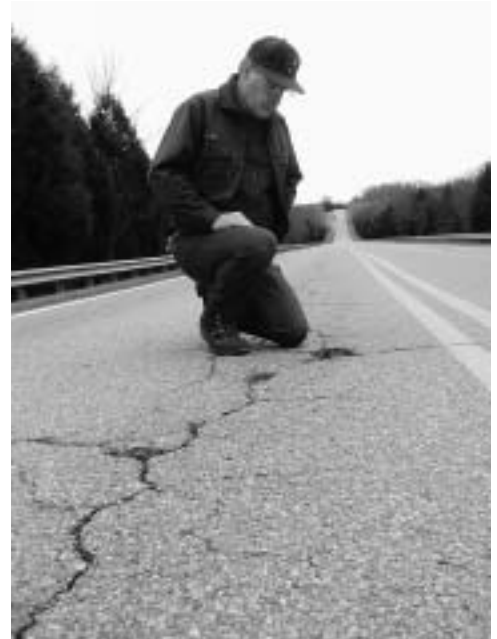
Roads Foreman Mark Davis examines damage in the park's roads.
