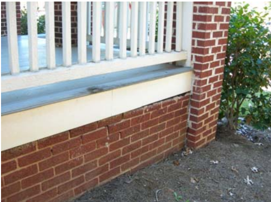
Porch foundation and pier of dissimilar brick and mortar
