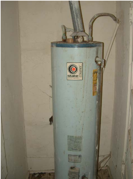
Water heater in Unit 4
