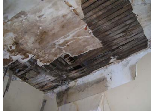
Damaged lath-and-plaster ceiling of first floor apartment unit.
