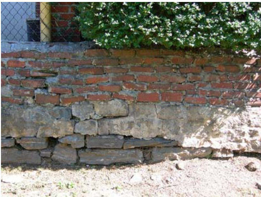
East retaining wall. Note deterioration of brick and mortar.
