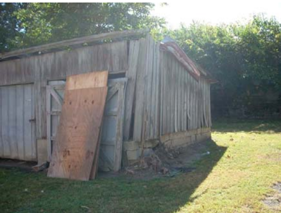
Northwest corner of garage. Note collapsed condition of foundation wall.
