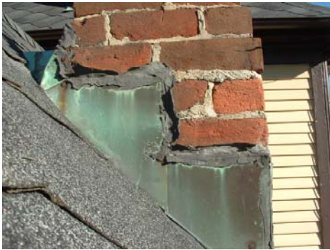
Deteriorated flashing sealant at kitchen chimney
