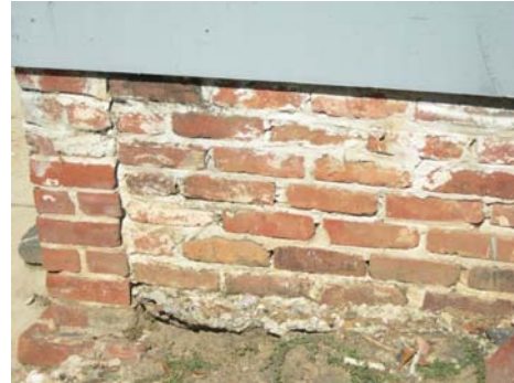
Poorly-constructed back porch foundation and pier
