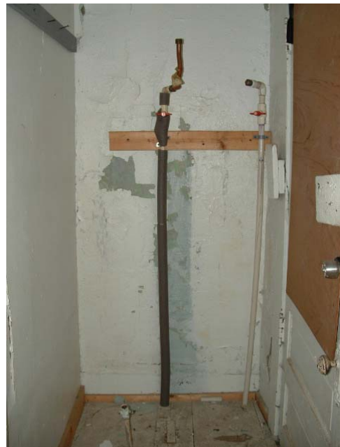
Typical installation for water heater in back hall utility room
