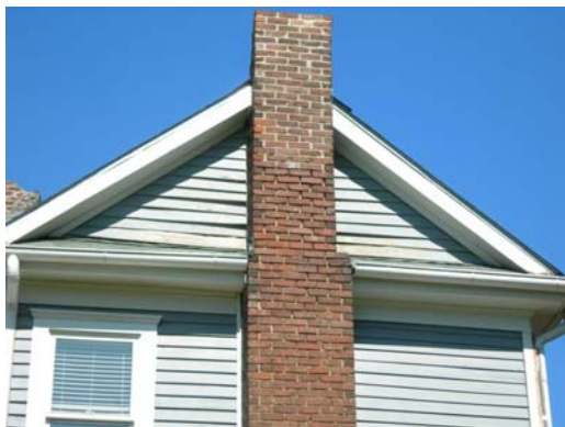
Inappropriate mortar repairs and missing mortar on south chimney
