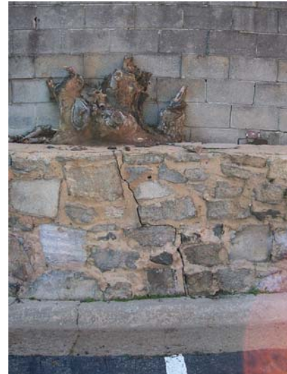
Tree stump growing out of retaining wall on south side property line, with stress cracks in lower wall
