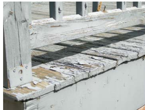
Deteriorated paint finish on back porch flooring and framing
