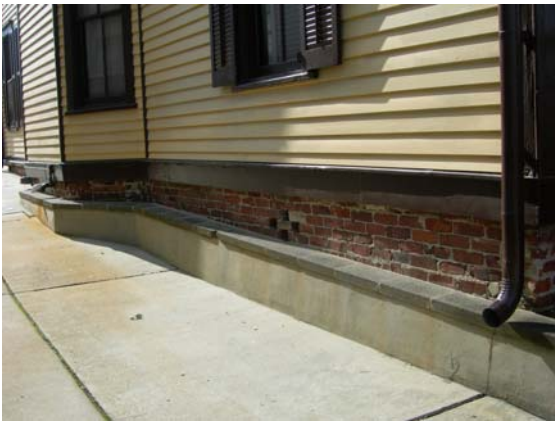
Retaining wall with gray concrete caps and continuous brick foundation on east elevation
