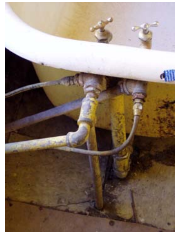
Typical water supply lines
