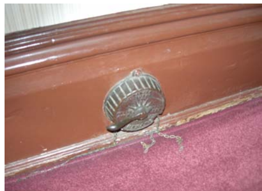
Manual furnace damper control in middle hall, first floor
