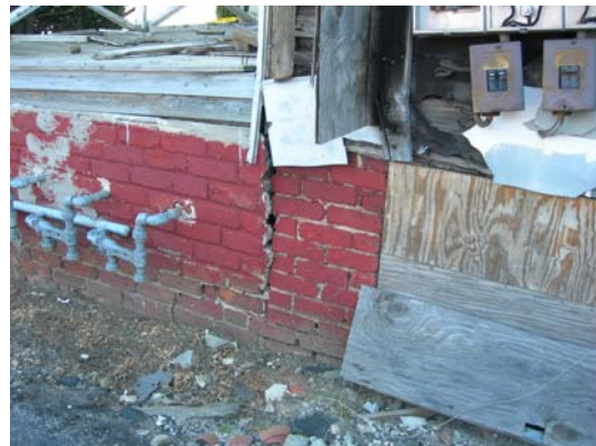
Failing porch foundation, west elevation
