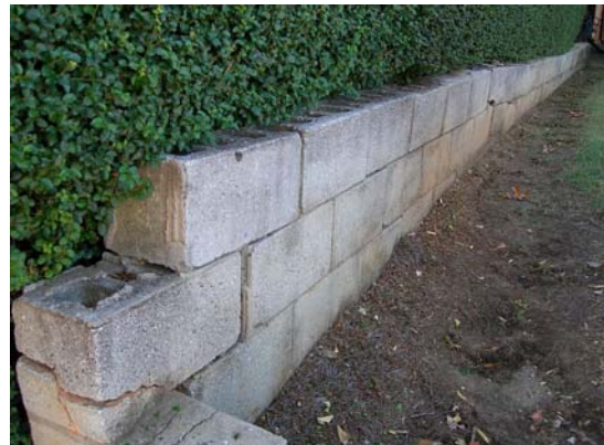
Cracked and damaged retaining wall along east boundary of lot
