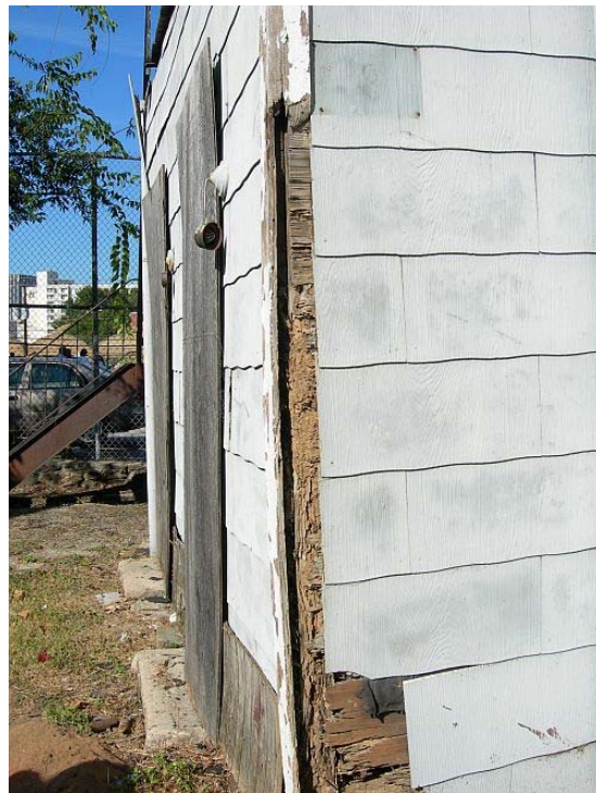
Missing cornerboard and damaged siding on south side of building
