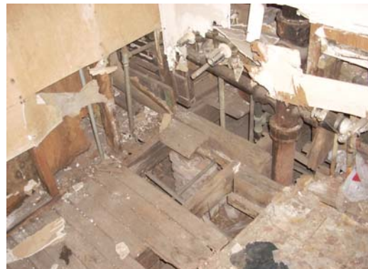
Typical deterioration of floor decking and walls near plumbing penetrations in Unit 3
