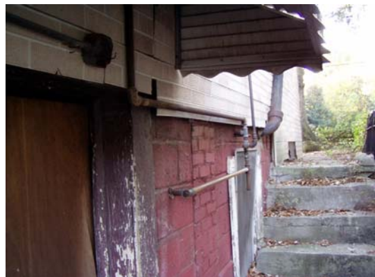
Water pipes, electrical conduit, and sanitary sewer piping surface mounted on the exterior, west elevation
