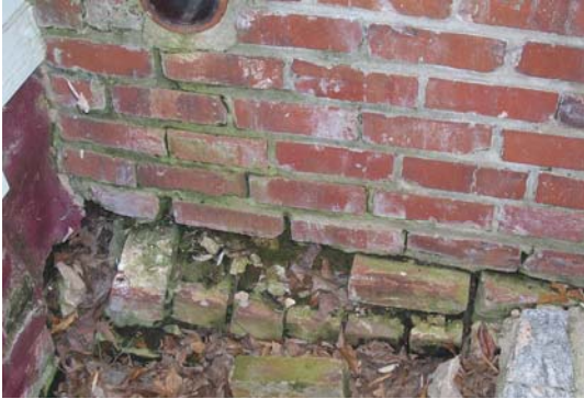
Detail of missing and detached bricks in west front retaining wall, north elevation
