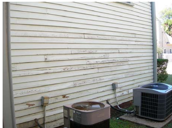
Air conditioning units at basement level of building, east elevation
