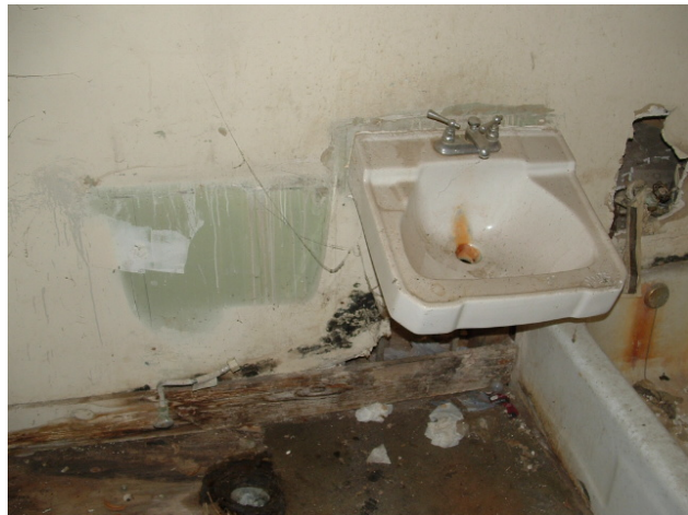
Bathroom fixtures in Unit 4
