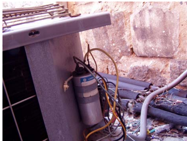
Condenser unit controls and damaged insulation
