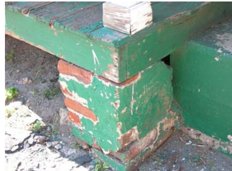
Deteriorated foundation pier
