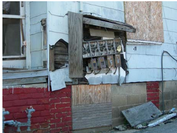
Remnant of former electrical box on west elevation
