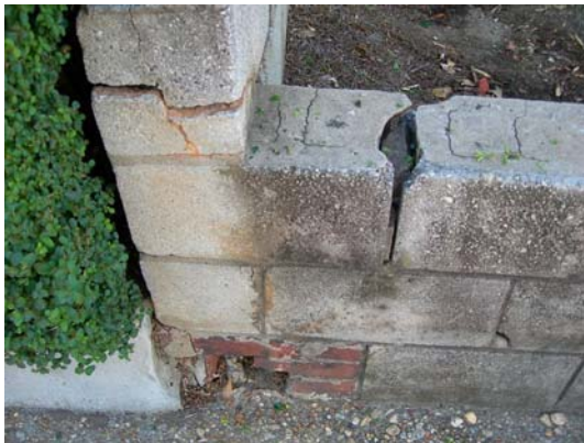
Cracked and deteriorating retaining wall at northeast corner of lot
