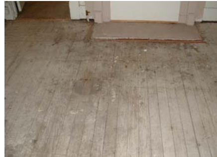
Typical flooring, hearth, and stub-up for gas pipe
