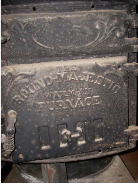
Original furnace in basement
