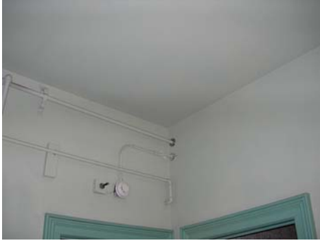
Peeling paint on kitchen ceiling is possibly the result of water damage
