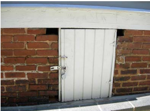
Basement entrance and missing and damaged brick and mortar, west elevation
