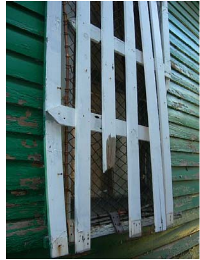
Broken picket of wood lattice over window on south elevation, 2008.
