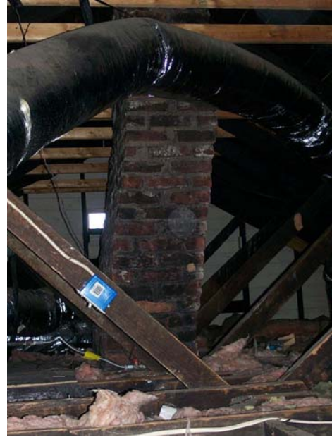
Chimney leans but does not appear to be unstable
