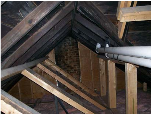
Stud-framed walls at rear chimney are not sealed to the chimney.
