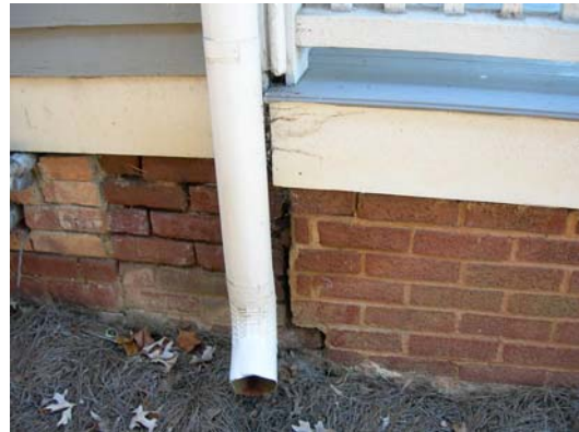
Separation of porch foundation from main building foundation
