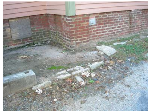
Partly-demolished retaining wall, brick infill between piers, and crawl space access on west elevation.
