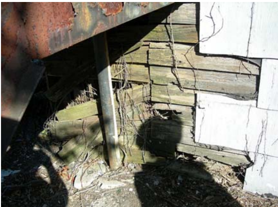
Metal stairway support and deteriorated composition siding over wood siding beneath back stairway
