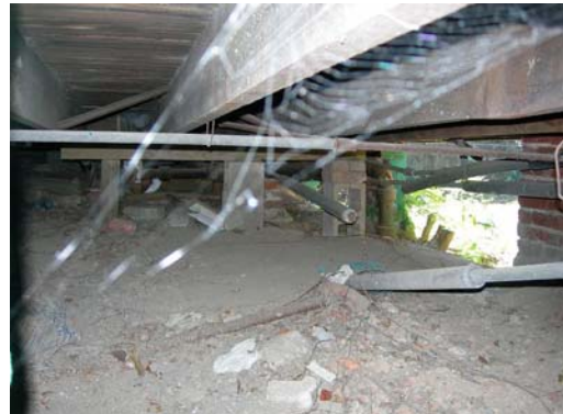
Assorted ad hoc floor supports beneath the building
