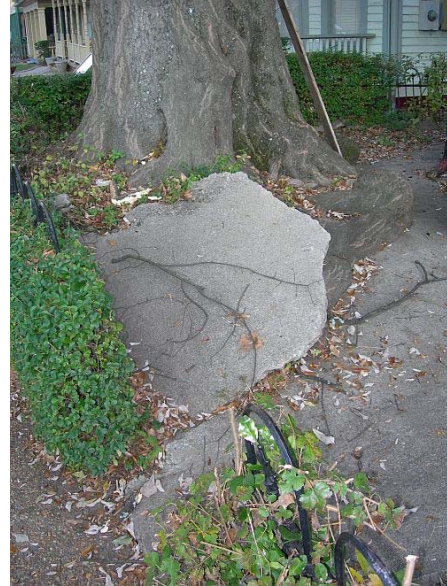
Growing tree has heaved the concrete sidewalk in the front yard
