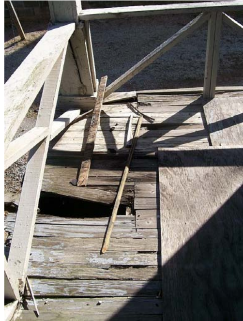
Pieced decking of front porch
