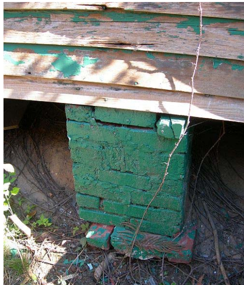
Typical support pier requiring repair
