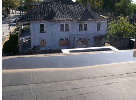
Ponding at east end of roof
