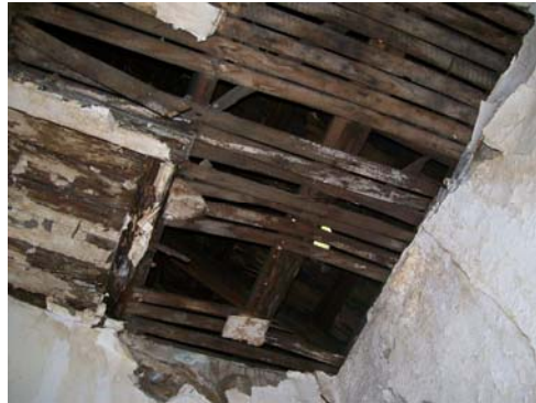
Typical damage to lath and plaster walls and ceilings
