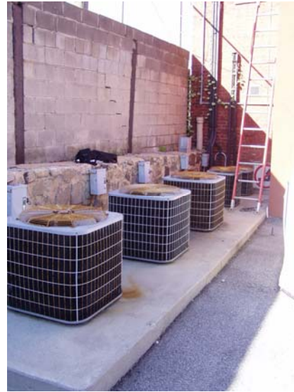
Fire Station condenser units
