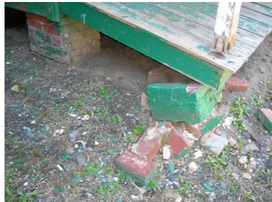
Failed porch piers and rotted porch posts on north side of front porch
