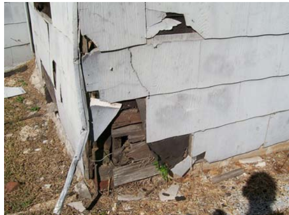
Damaged siding, underlying sheathing, and corner boards
