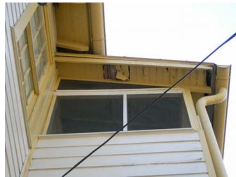
Paint deterioration underside of west porch roof
