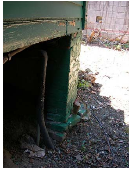
Northwest pier is leaning, missing bricks, and has a tree growing out of it
