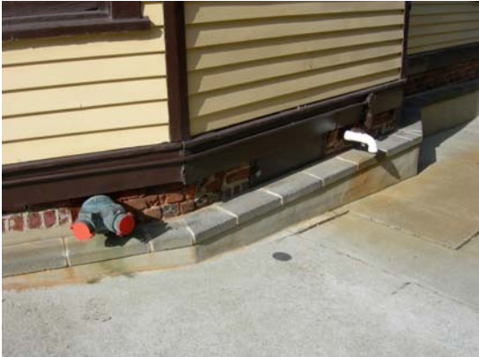
Metal-covered access hatch to partial basement blocked by concrete retaining wall on east elevation
