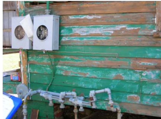
Gas and electrical utilities on north side of building
