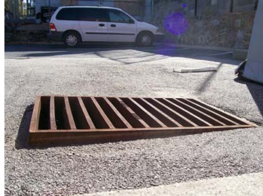
Drainage grate in east parking lot is improperly set
