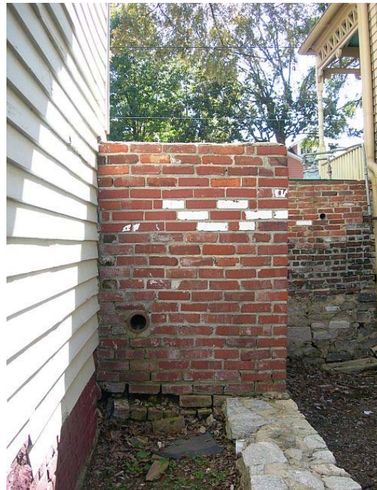
Brick retaining wall with drain pipe and stone retaining wall on west side of building
