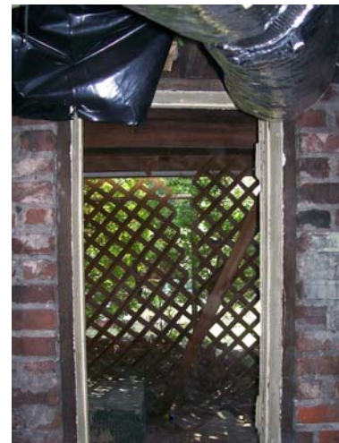
Additional bracing needed over crawl space door
