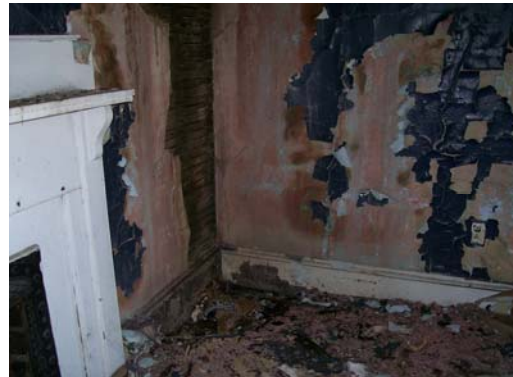
Moisture damage to plaster walls on second floor
