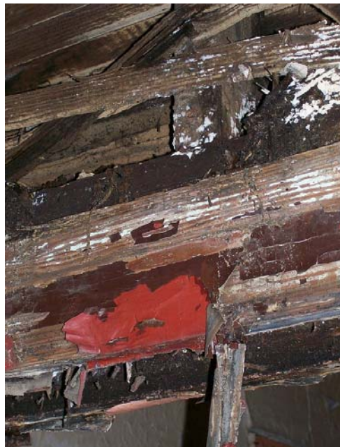
Rotted framing members in attic area
