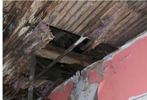
Failed lath and plaster ceiling
