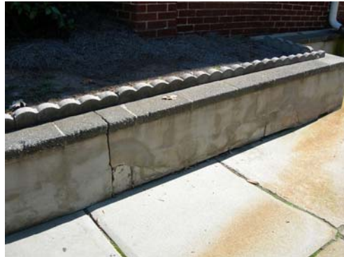
Cracking in retaining wall along west side of building
