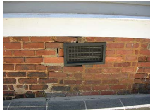
Basement vent, with inappropriate and failing repairs to foundation wall
