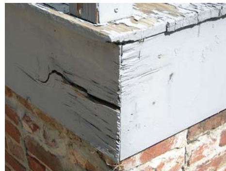
Deteriorating back porch flooring and framing
