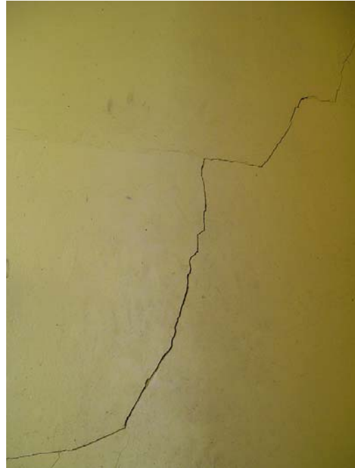
Stress crack in upstairs bathroom
