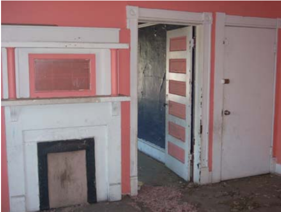
Fireplace surround and mantel, original and replacement doors, original wood trim in Unit 491-1/2
