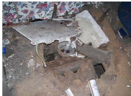
Damaged flooring at sanitary pipe
