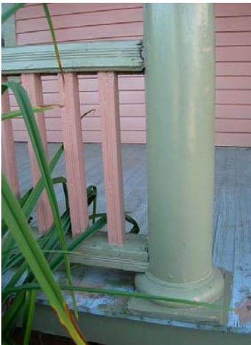
Deteriorated railing to column connection on front porch
