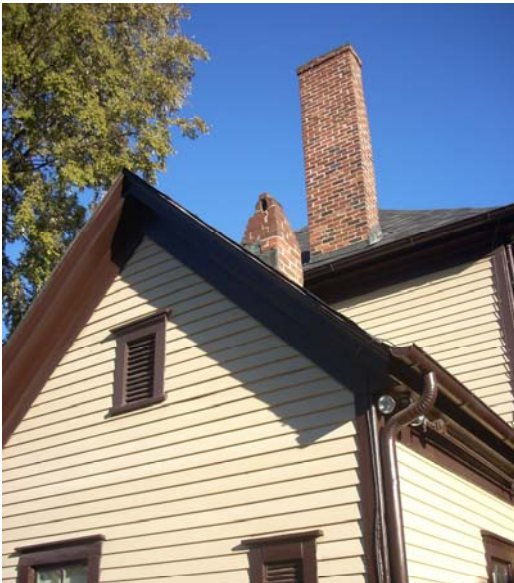
Detail of chimneys on rear east side of building and louvered openings on south elevation of rear projection
