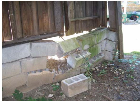
Northwest foundation is near collapse
