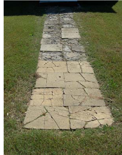
Deteriorated walkway of concrete pavers to back stairs
