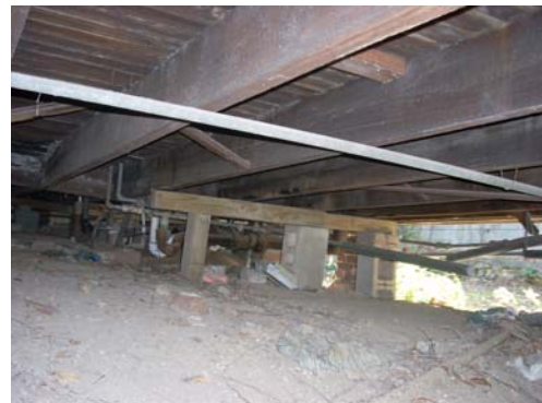
Temporary support beneath west end of building is not adequate
