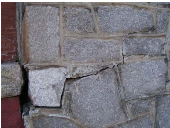
Stress cracks in retaining wall at southwest corner of building
