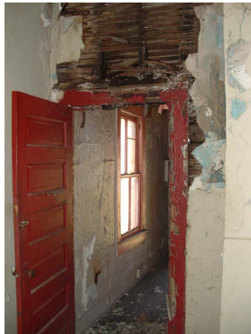
Typical wall and ceiling deterioration
