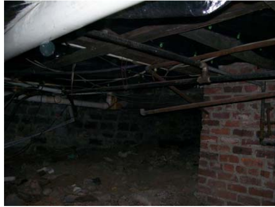
Pipe hanging loose in the crawlspace
