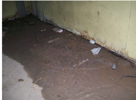
Mud pit and mold accumulating in basement
