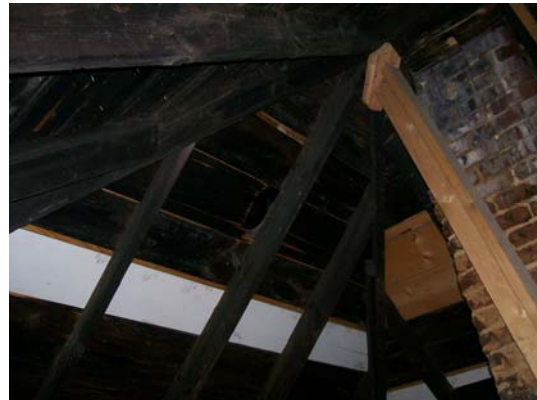
Additional bracing for roof rafters and replacement roof decking
