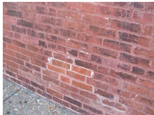
Inappropriate brick and mortar replacement
