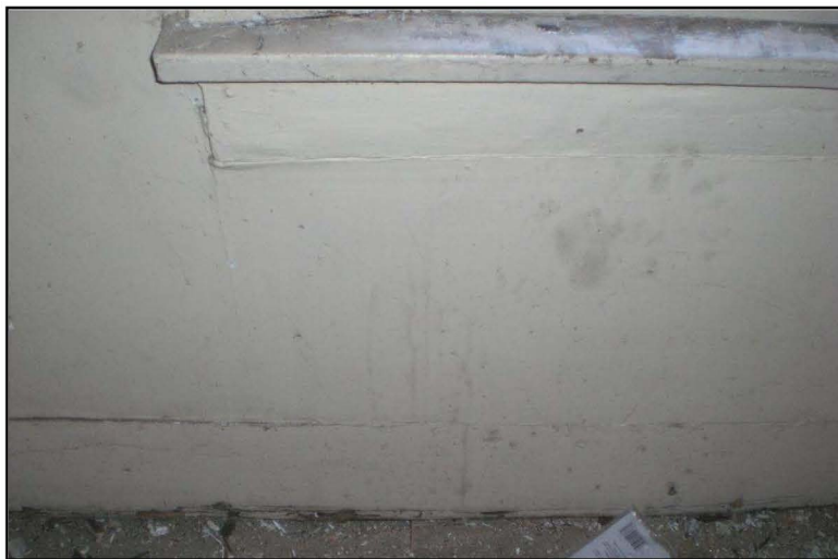
Figure 23 – Improper plaster repair, room 108, west wall (courtesy Rosemary Davis)
