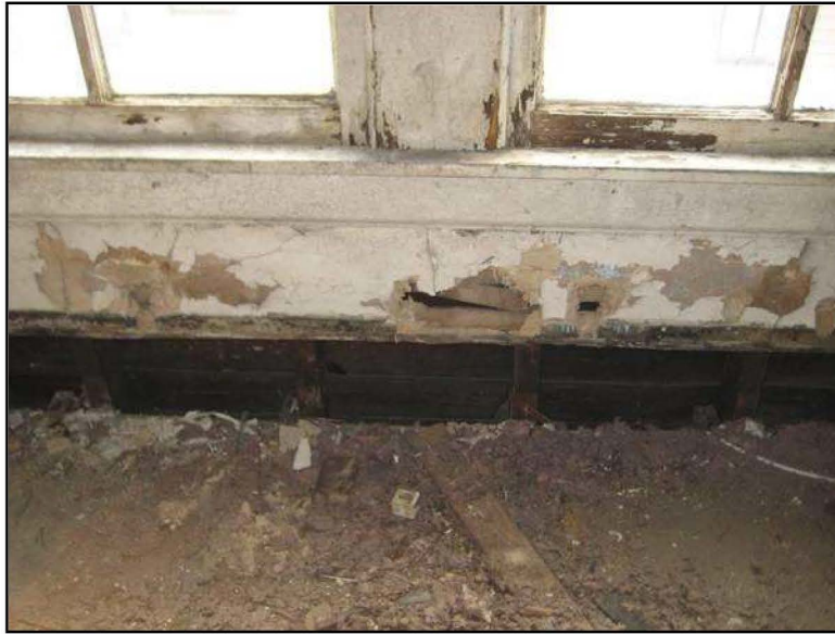
Figure 21 – Non-existent baseboard in room 203, east wall
