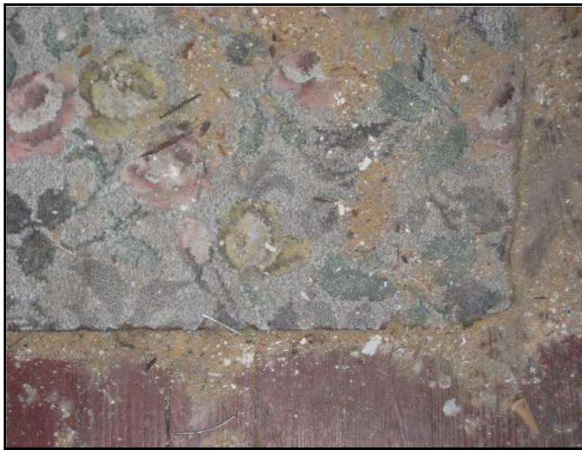
Figure 7 – Detail of vinyl in room 201
