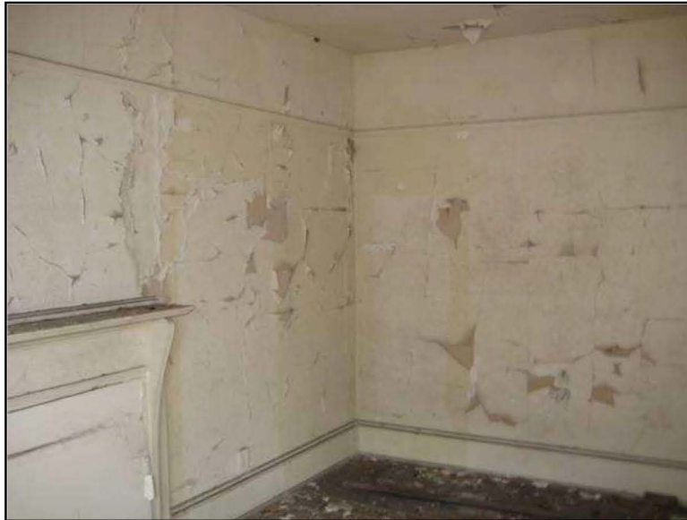
Figure 18 – Peeling plaster in room 203, southwest
