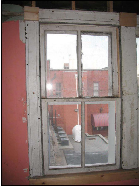
Figure 24 – Inappropriate corner blocking, room 208, west wall (courtesy Angelica Dion)
