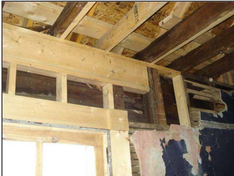
Figure 5 – Example of repairs by NPS in room 207, west wall (courtesy of Holly Schwarzmann)
