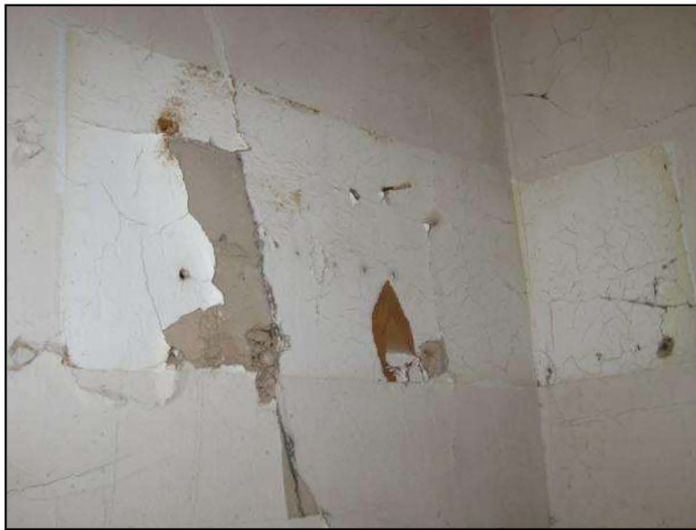
Figure 13 – Room 204 ghosting from cabinets, southeast wall
