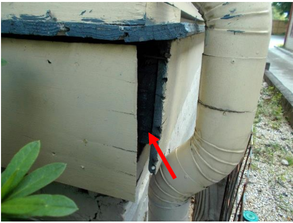
FIGURE 57. Open joint and displacement of wood porch apron.
