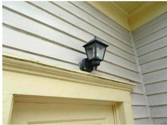
FIGURE 27. Non-original sconce above exterior door at south elevation.
