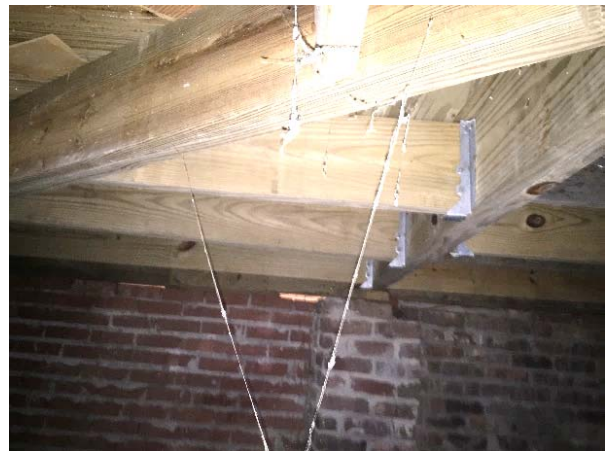
FIGURE 98. Floor joists with joist hangers at porch flooring.
