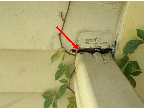
FIGURE 58. Open joint and displacement at balustrade rail.
