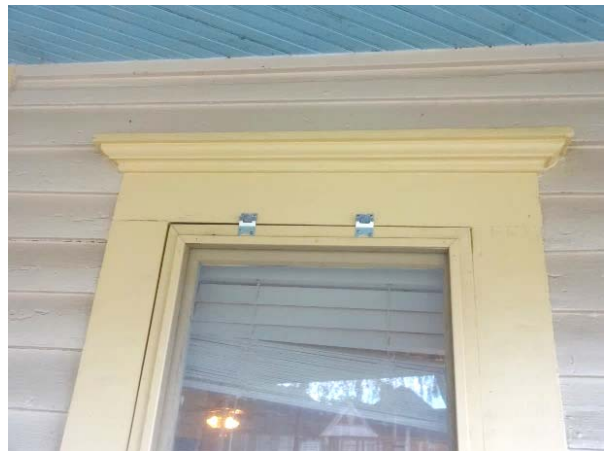
FIGURE 40. Crown molding header casing at window openings. Also note metal hooks for window screens.
