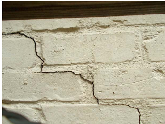
FIGURE 45. Step cracking at the brick foundation wall.
