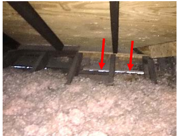
FIGURE 104. Large air gaps between roof and wall framing.
