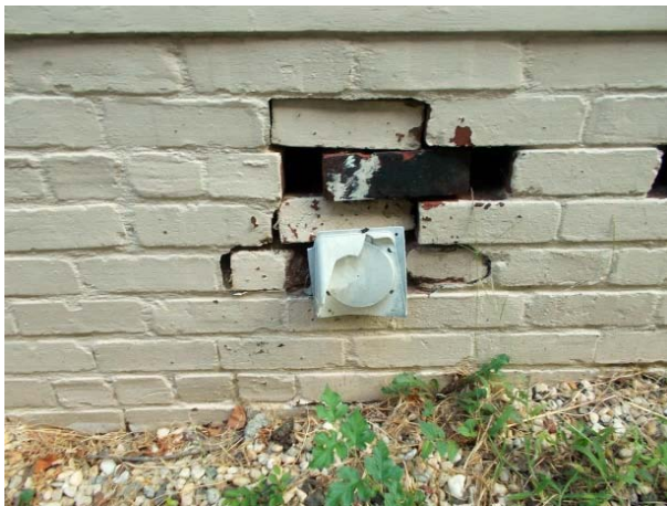
FIGURE 48. Displaced brick associated with previous alterations to the brick masonry.
