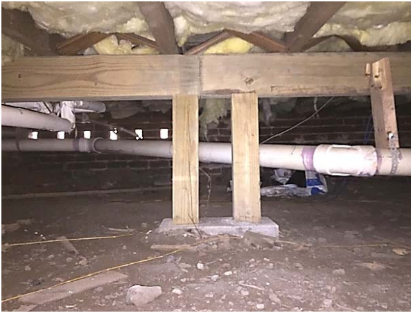
FIGURE 113. PVC waste lines in crawl space.
