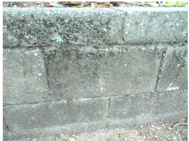
FIGURE 51. Organic growth on CMU at retaining wall.
