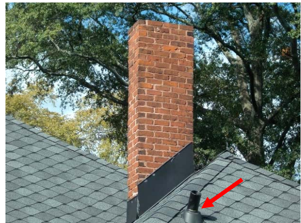
FIGURE 43. Brick masonry chimney with sheet-metal flashing. Also note vent pipe near base of chimney (arrow).
