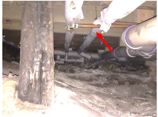
FIGURE 24. Pipes of various kinds suspended from metal straps attached to floor joists.
