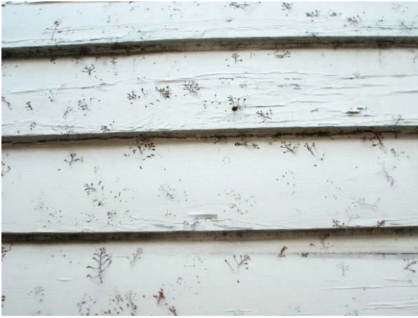
FIGURE 63. Tendrils from previously existing vegetation are attached to siding.
