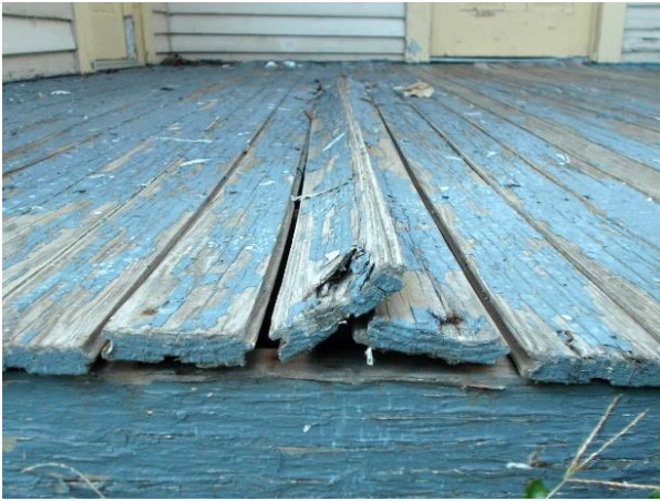
FIGURE 59. Twisting and buckling of wood decking at front porch.
