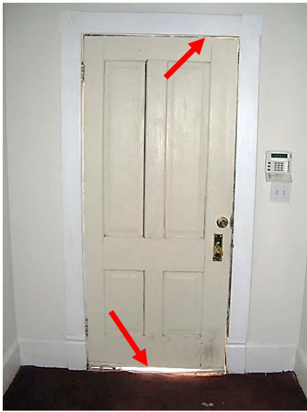
FIGURE 88. Non-original rear exterior door. Note deteriorated threshold and gaps around door.
