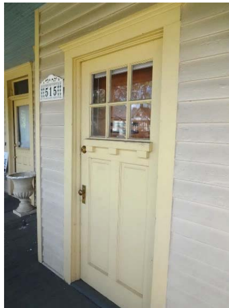
FIGURE 33. Door opening at west end of north elevation has been fixed in place.
