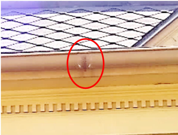
FIGURE 67. Loose and displaced gutter strap.
