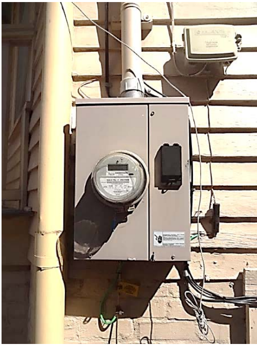
FIGURE 110. Electric service meter base and telecommunications box.
