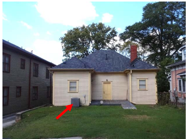
FIGURE 108. New split system condensing unit.
