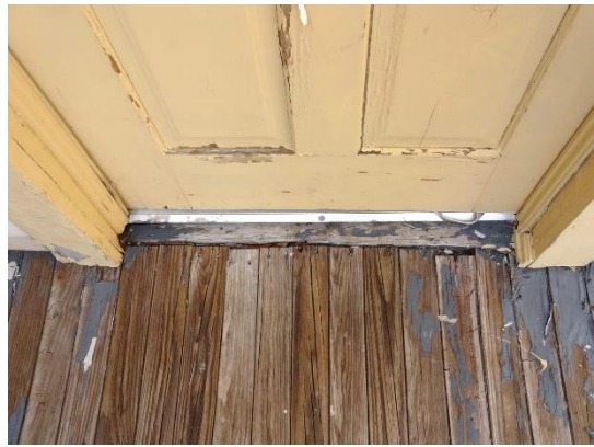
FIGURE 61. Peeling and debonding of paint on wood decking at rear patio.
