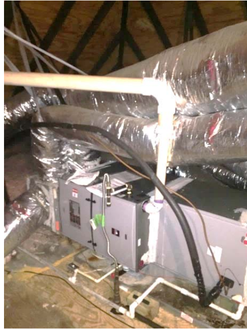
FIGURE 107. New heating and air conditioning unit in the attic.
