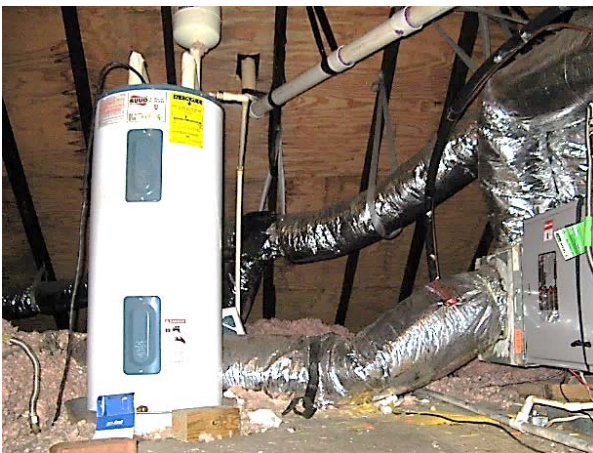
FIGURE 114. Gas water heater in the attic.
