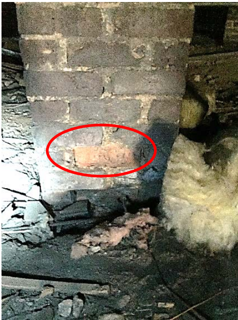
FIGURE 106. Spalling of brick and masonry foundation piers.
