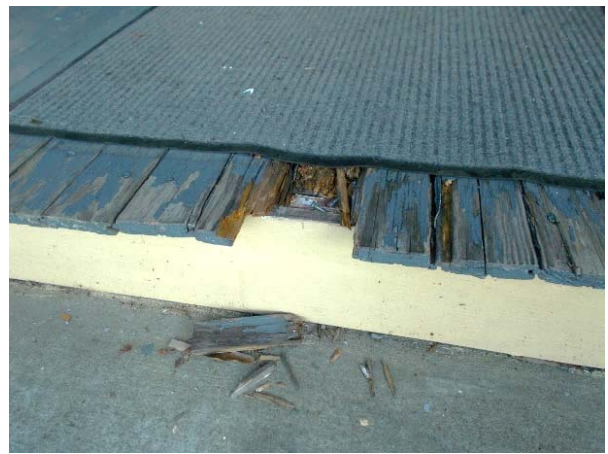
FIGURE 55. Deteriorated wood decking at front porch.
