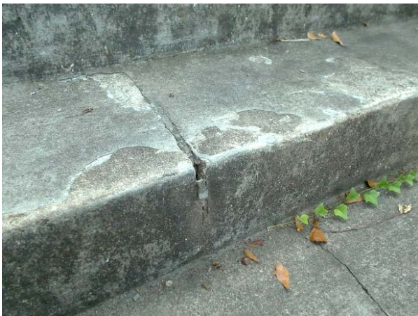
FIGURE 52. Cracking of the concrete at stairs.
