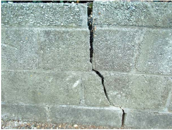
FIGURE 46. Step cracking at the CMU retaining wall.
