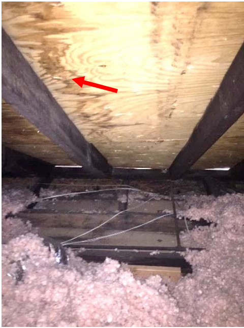
FIGURE 105. Moisture staining on plywood sheathing.
