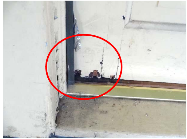
FIGURE 64. Deteriorated wood at bottom stile of the wood door.
