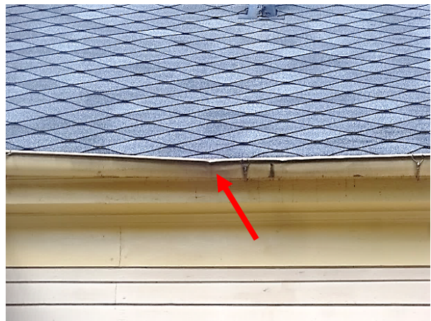
FIGURE 68. Damaged gutter at south elevation of the building.
