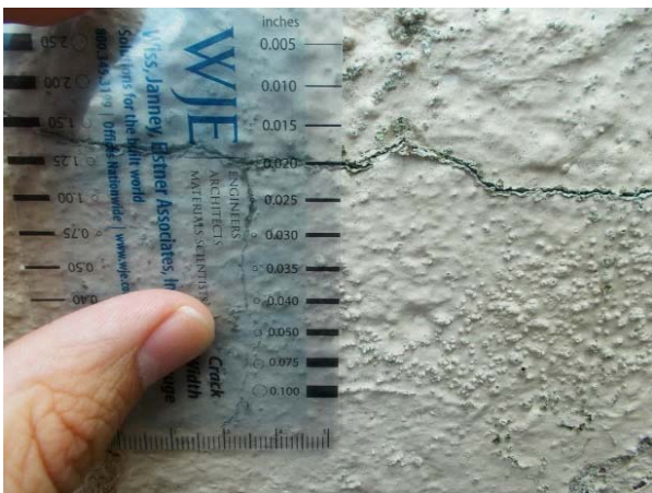
FIGURE 53. Hairline cracking at concrete coping units at cheek walls.
