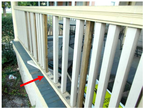
FIGURE 62. Balustrade at north porch with missing spindles.
