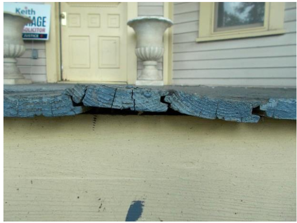
FIGURE 60. Mild cupping of floor decking at front porch.
