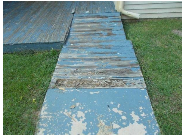
FIGURE 56. Deteriorated wood decking at rear patio.
