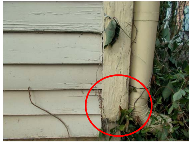
FIGURE 54. Deteriorated wood trim. Note that deterioration is more significant at bottom of trim.
