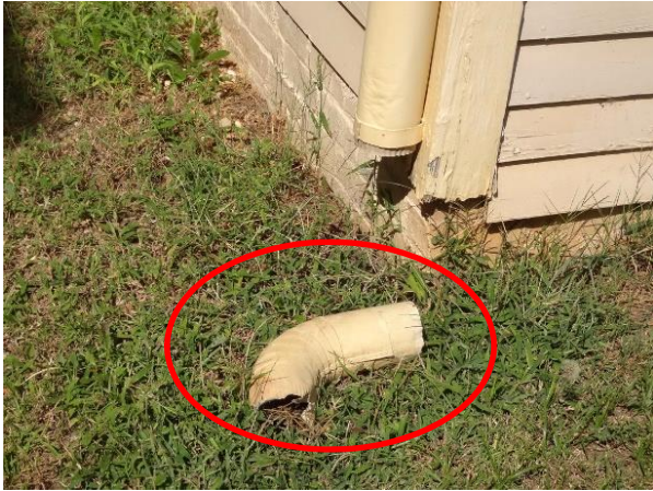
FIGURE 66. Disconnected leader at northwest corner of the building.
