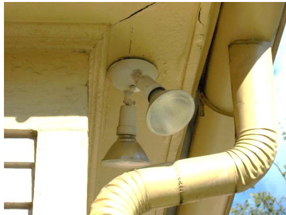
FIGURE 28. Flood light mounted to underside of roof eave.
