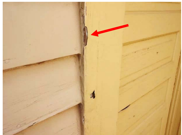
FIGURE 65. Deteriorated paint at wood trim and door leaf.
