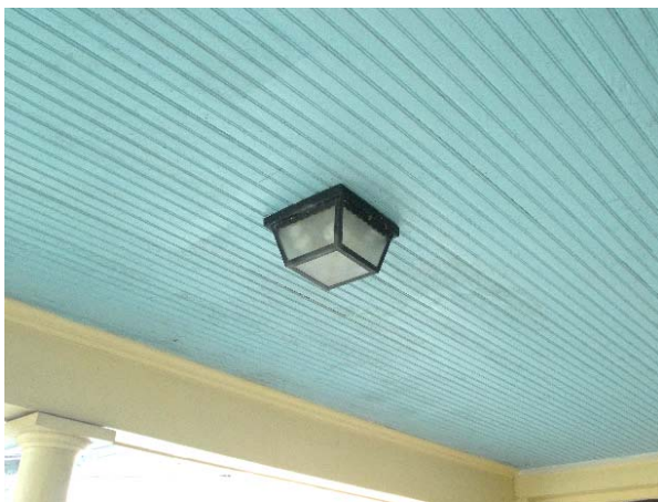
FIGURE 29. Surface-mounted light fixture at ceiling of north porch.
