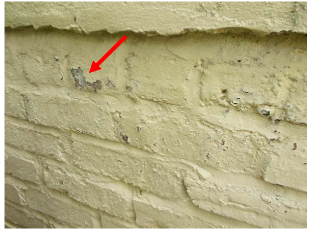
FIGURE 50. Peeling paint at brick foundation walls.
