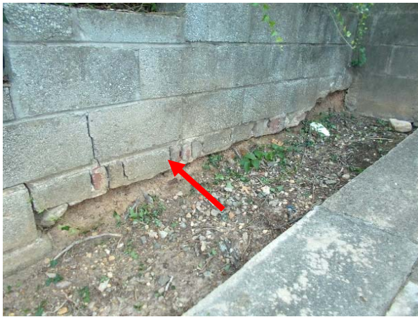
FIGURE 47. The foundation at the west side of the retaining wall has been undermined.
