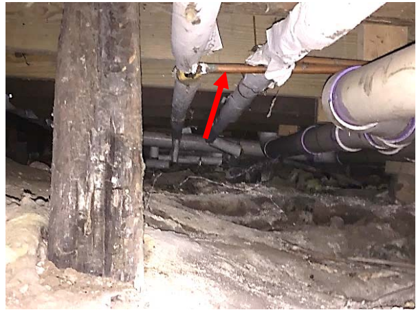
FIGURE 112. Missing insulation on copper water pipes in the crawl space.
