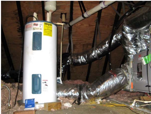
FIGURE 109. Gas water heater in the attic.
