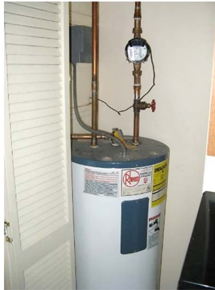
FIGURE 147. Typical electric hot water heater at second-floor apartment.
