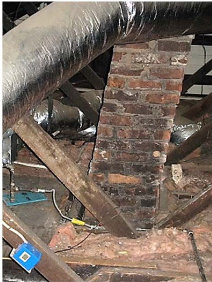
FIGURE 114. Curvature at chimney.
