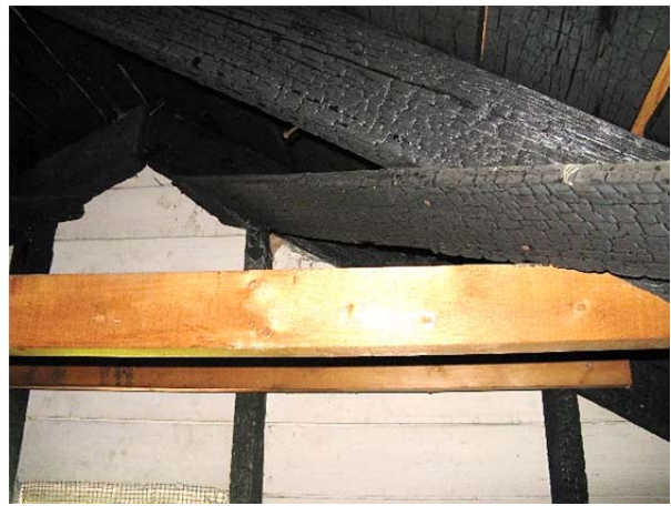
FIGURE 133. Severe fire damage at diagonal cross bracing at north end gable roof framing.
