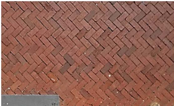
FIGURE 11. Brick sidewalk paving along east elevation of the building. Paving set in a herringbone pattern.
