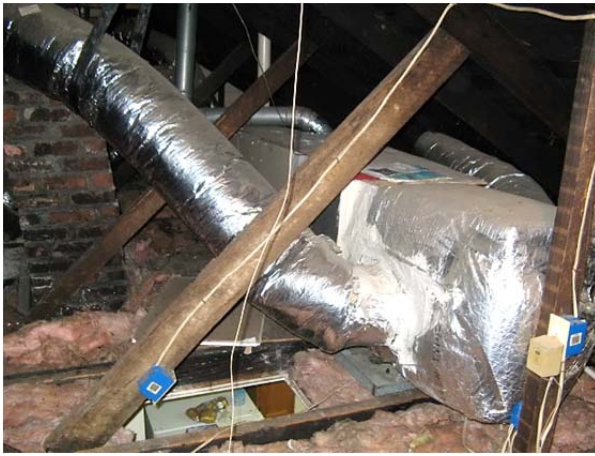
FIGURE 140. Forced air furnace in attic.
