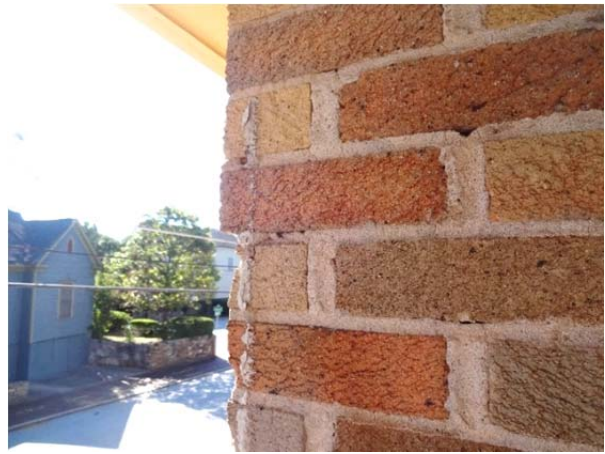
FIGURE 61. Remnants of sealant from previously removed screen wall at front entrance porch.
