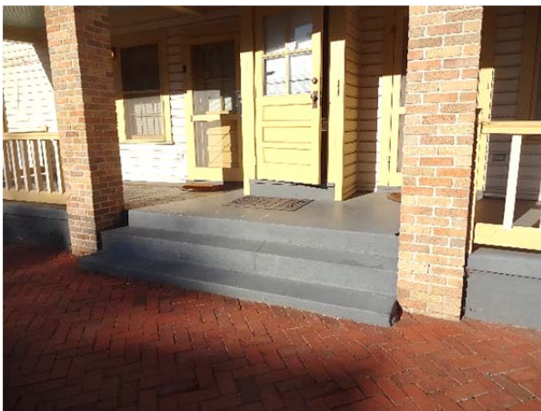
FIGURE 27. Brick foundation with cementitious parge coating and concrete deck slab at front entrance porch.
