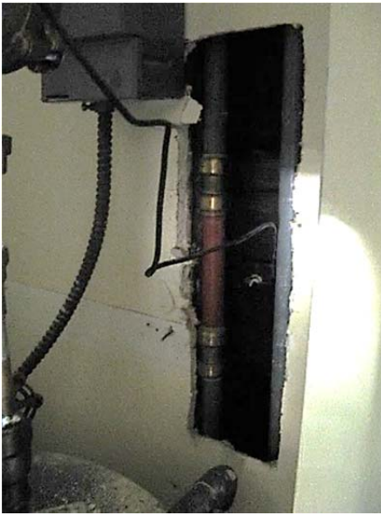
FIGURE 137. Opening in gypsum wall board at hot water heater, north second-floor apartment.
