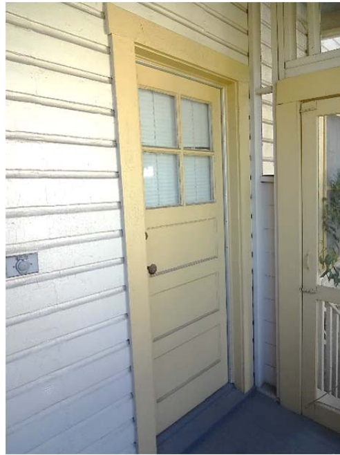
FIGURE 39. Wood-framed exterior doors at the west elevation of the building differ slightly from typical doors on the east elevation.
