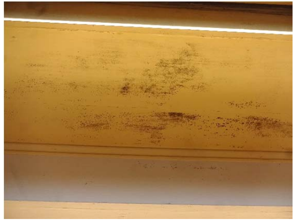
FIGURE 69. Biological growth on the underside of box beams at the front porch.
