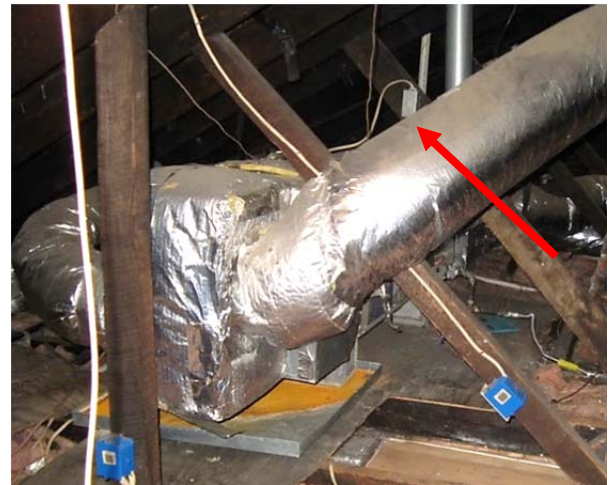
FIGURE 135. Toggle switch for HVAC unit.
