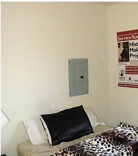
FIGURE 139. Electrical panel above bed at north apartment.
