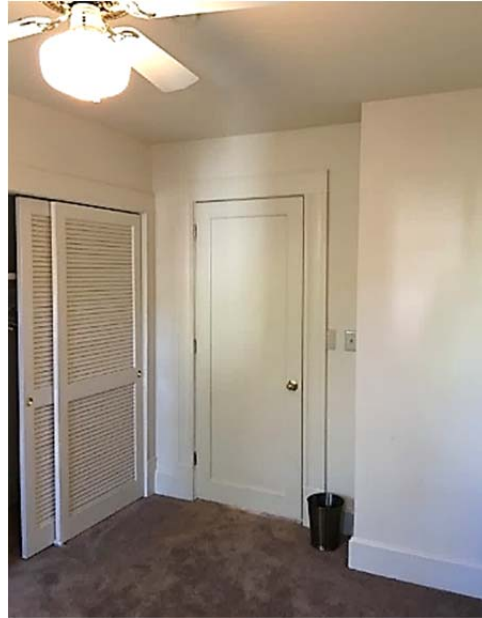
FIGURE 101. Interior bedroom door to living room (center) and sliding closet doors (left).
