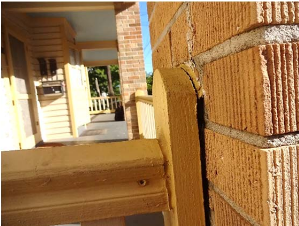
FIGURE 68. Displacement and open joints at vertical trim boards.
