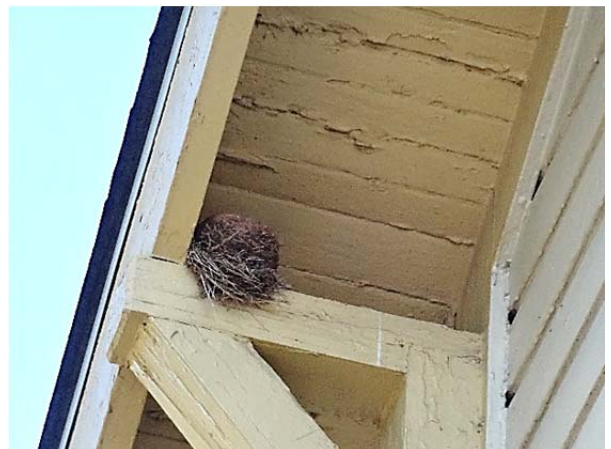
FIGURE 74. Bird's nest at roof bracket and eave.
