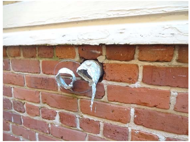
FIGURE 143. Flexible foil exhaust vent from first-floor bathroom at penetration of south skirt wall.
