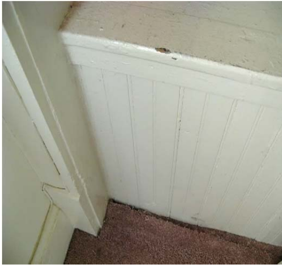
FIGURE 105. Beaded wood paneling in the closet above the north stair appears original.
