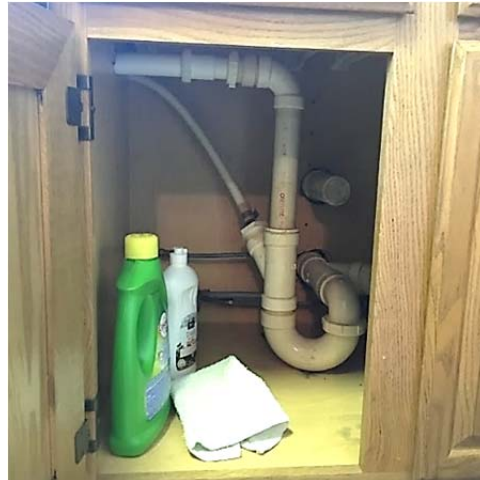
FIGURE 148. Drain piping below kitchen sink at first-floor apartment.
