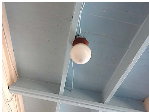
FIGURE 34. The first-floor ceiling of the enclosed rear porch. Note exposed framing and lighting.
