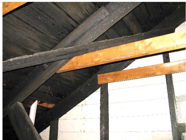
FIGURE 134. Fire damage observed at wood rafters at north end of roof.
