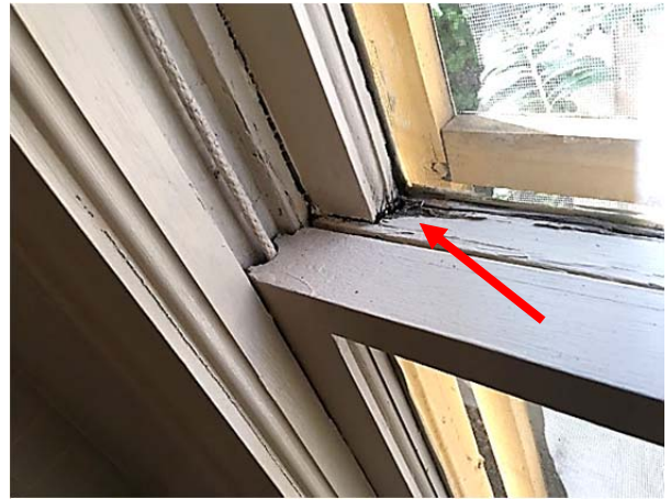
FIGURE 121. Moisture damage at interior of window sash.
