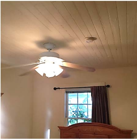
FIGURE 78. An original wood-panel ceiling with crown molding remains in the south bedroom of the lower unit.
