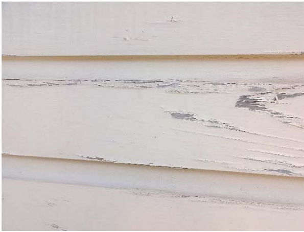
FIGURE 71. Peeling paint at wood siding.
