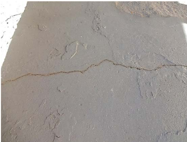
FIGURE 63. Untreated crack in concrete deck at front porch.
