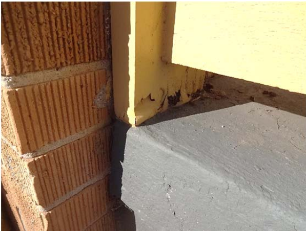
FIGURE 66. Deteriorated wood adjacent to brick piers and concrete decking at front porch.
