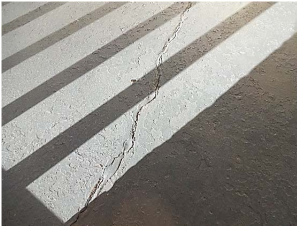
FIGURE 62. Previously repaired crack in concrete deck at front porch deck has failed.
