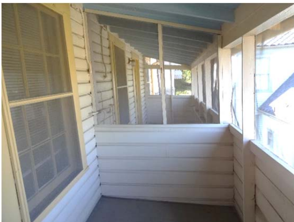
FIGURE 36. Wood-framed partition wall that separates the north and south ends of the rear porch at the second-floor level.
