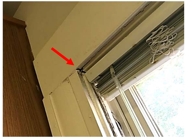
FIGURE 122. Separation of components at interior of window.
