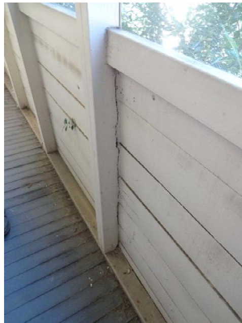
FIGURE 33. Enclosed rear porch interior walls consist of shiplap siding and mesh screening fastened to framing members.
