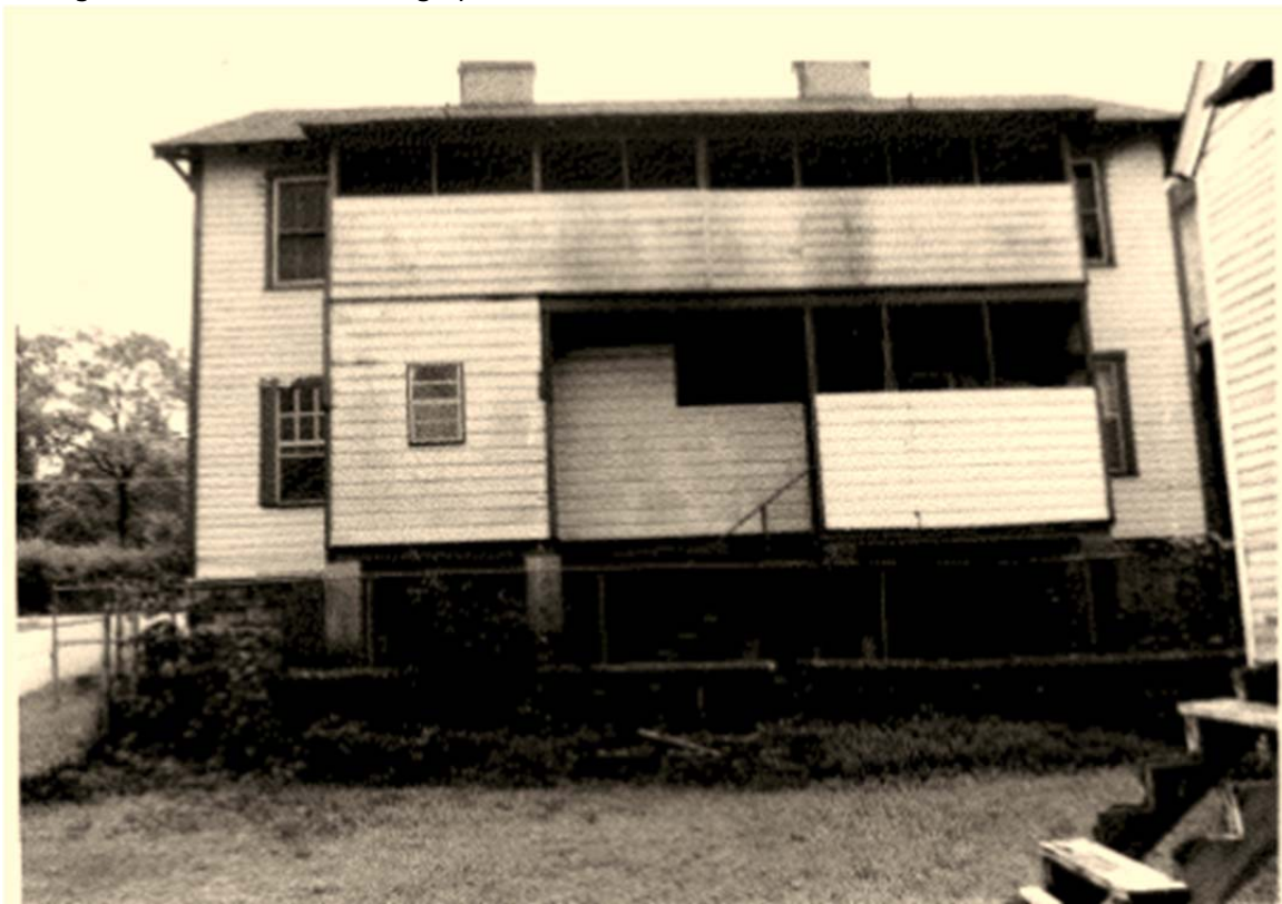
FIGURE 8. 54 Howell Street, rear, west, facade, after the 1985 fire showing what appears to be only smoke damage. (Source: Division of Facilities Management, 1981-1991 - Photographs)
