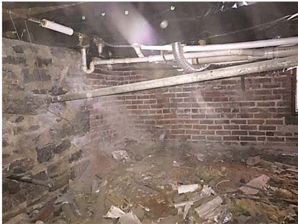
FIGURE 145. Drain and supply piping at crawl space.
