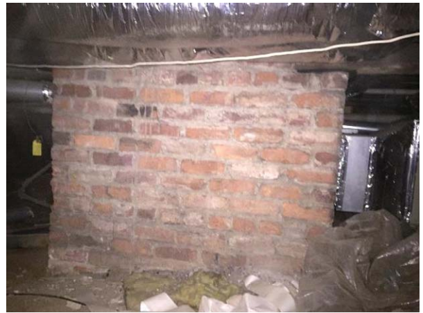
FIGURE 21. Brick masonry chimney foundation.
