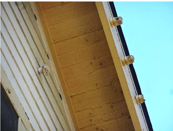
FIGURE 48. Underside of the eaves with the wood plank decking exposed to view.
