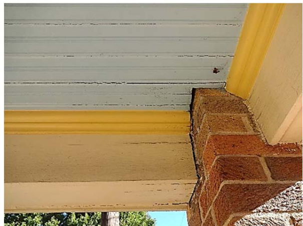
FIGURE 70. Open and displaced bead boards at the first-floor ceiling of the front porch.
