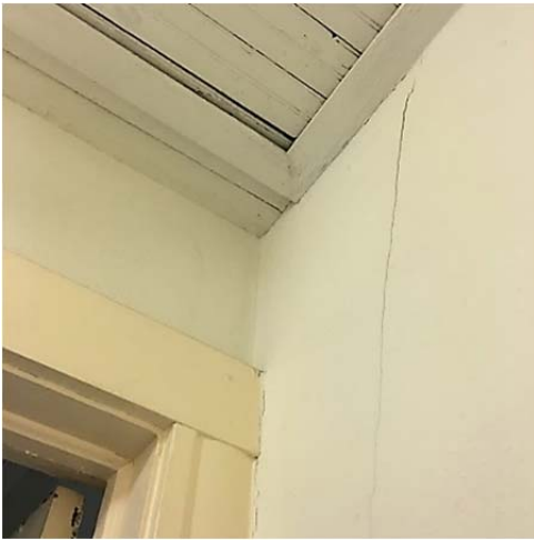
FIGURE 116. Linear crack in plaster at rear stair.
