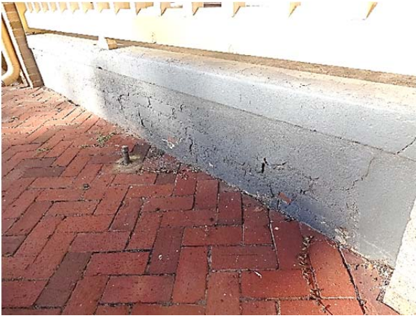
FIGURE 58. Debonded parge coating at front porch foundation.
