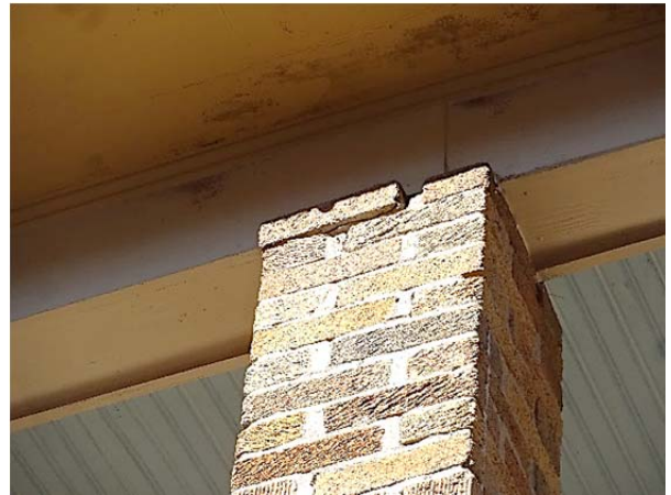
FIGURE 57. Displaced brick unit at top of pier.
