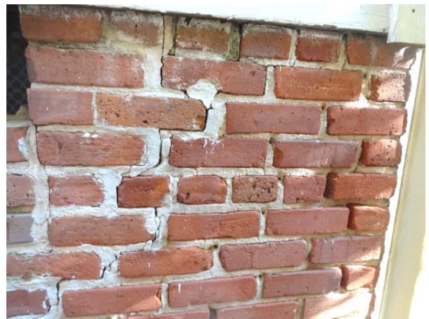
FIGURE 56. Open and exposed joints are located at brick masonry foundation wall.
