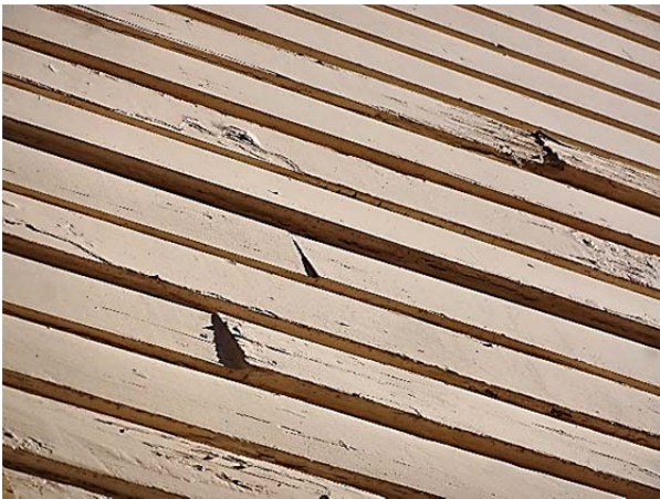
FIGURE 67. Twisting of wood cladding was most pronounced the ends of the boards.
