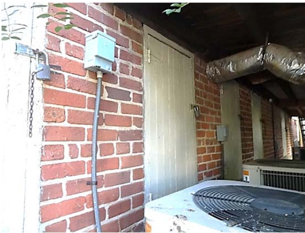
FIGURE 142. A/C condensing units under the rear porch.
