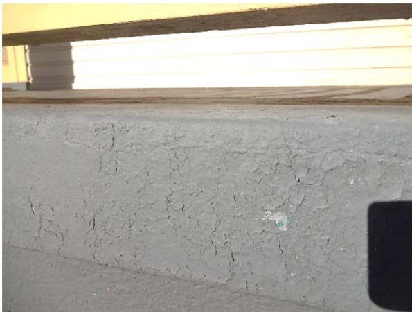
FIGURE 64. Peeling and flaking paint on concrete at front porch.
