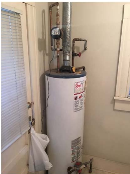
FIGURE 146. Gas hot water heater at first-floor apartment (located in laundry).
