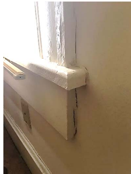
FIGURE 115. Typical separation between trim elements and gypsum board.
