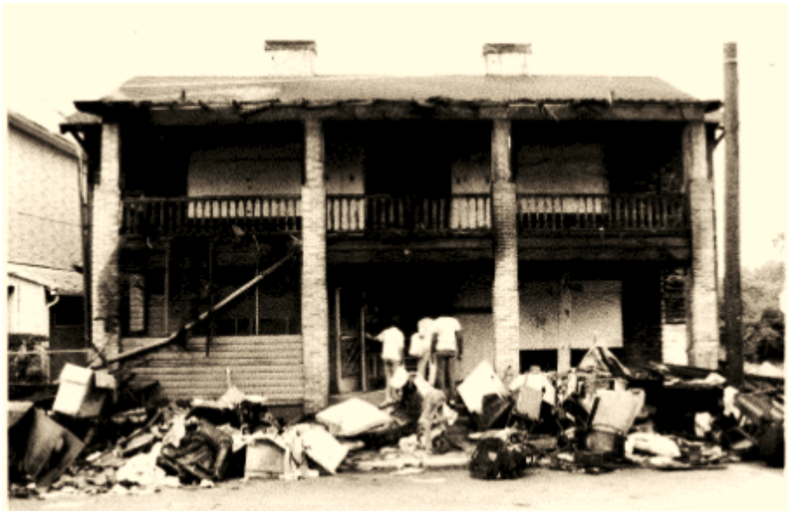
FIGURE 7. 54 Howell Street, front, east, facade after the 1985 fire. (Source: Division of Facilities Management, 1981-1991 – Photographs)
