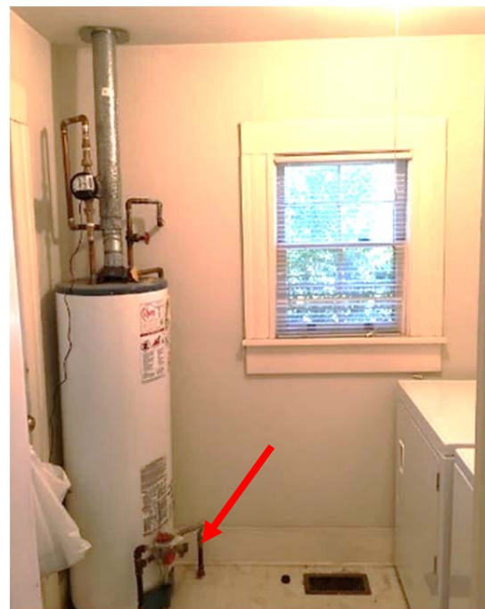
FIGURE 136. Floor penetration of gas service line at laundry hot water heater. Water supply piping entering wall is uninsulated.
