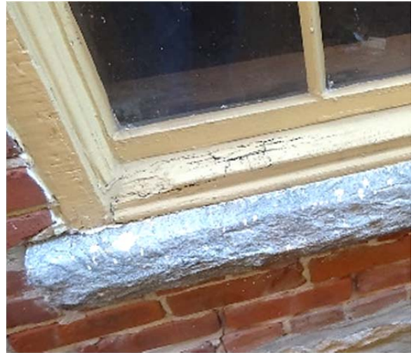
FIGURE 73. Deteriorated and decayed wood at basement windowsill.
