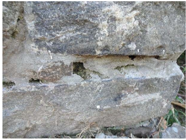
FIGURE 60. Biological growth at joints in foundation wall.
