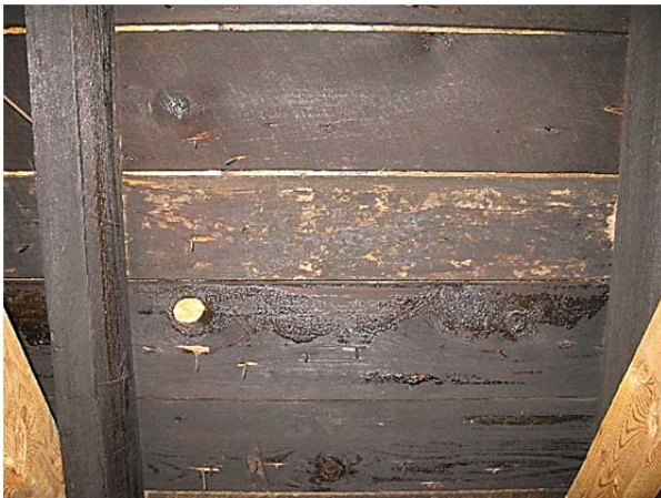
FIGURE 128. View of wood plank roof sheathing. Note plywood sheathing applied over plank.
