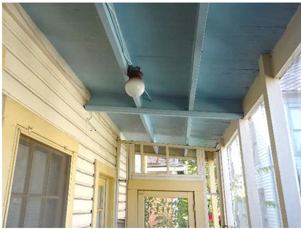
FIGURE 131. Wood framing for second floor of rear porch is exposed to view.
