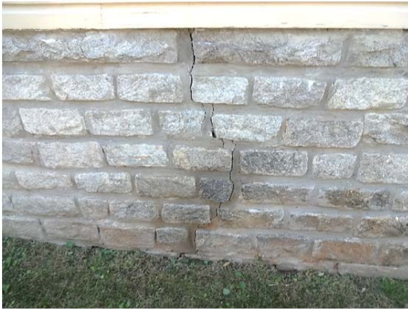
FIGURE 53. Vertical cracking and moisture staining at stone foundation wall.
