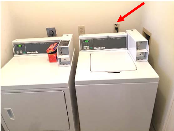
FIGURE 138. Broken face plate at washer receptacle adjacent to washing machine water and drain outlet box.
