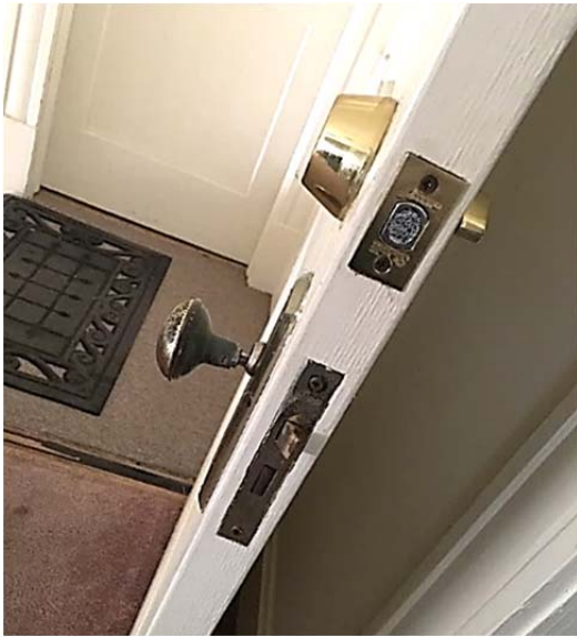
FIGURE 118. Typical non-original hardware at entrance doors. Knobs are loose and / or missing due to wear and deterioration.
