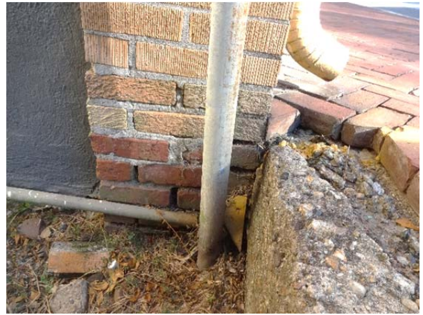
FIGURE 55. Open and exposed joints are located at brick masonry pier.
