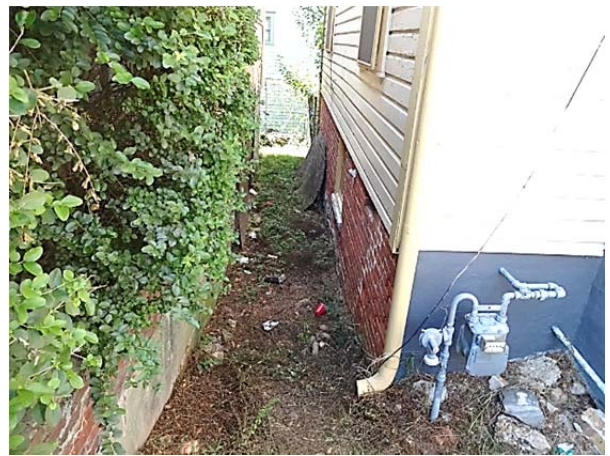
FIGURE 144. Gas meter at southeast corner of building (service from Howell Street).
