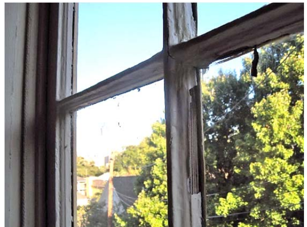
FIGURE 123. Paint delamination at muntin.
