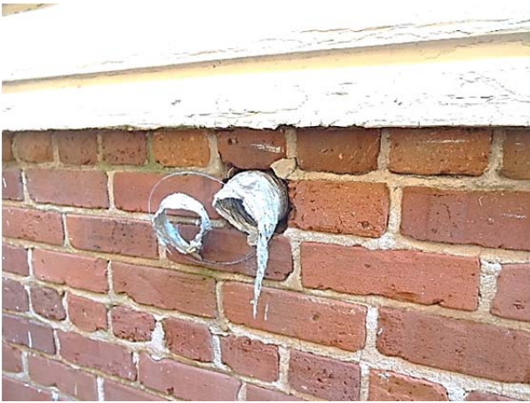
FIGURE 59. Non-original penetration at brick foundation wall.
