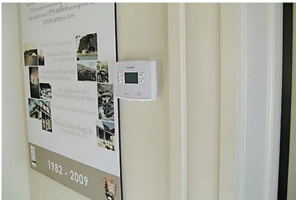
FIGURE 141. Typical digital thermostat in living room.
