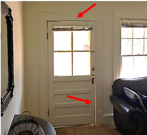
FIGURE 119. Air gaps at perimeter of exterior door.
