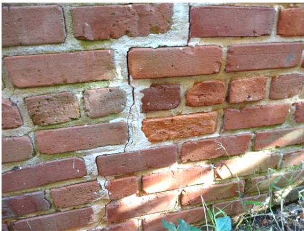
FIGURE 54. Vertical cracking at brick foundation wall.
