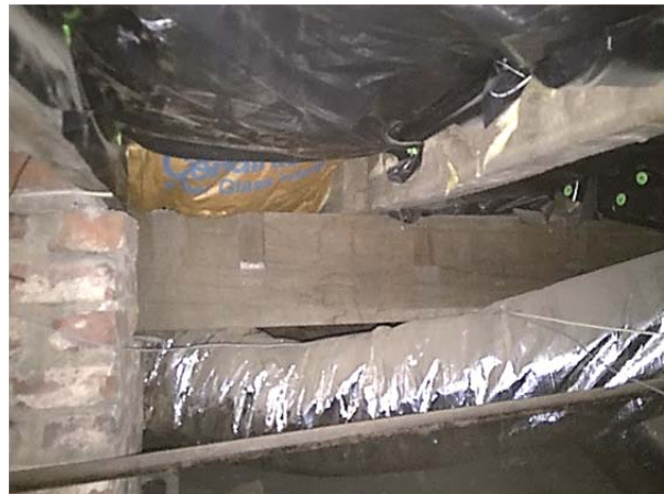
FIGURE 125. View of floor joists. Pocket between joists has been filled with batt insulation.
