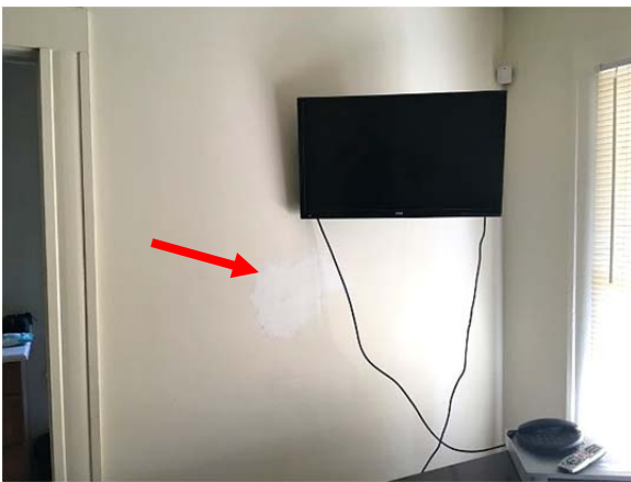
FIGURE 117. Patch at living room wall.
