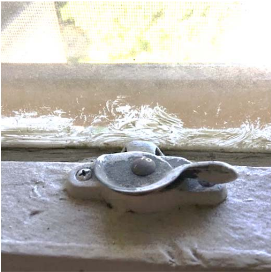
FIGURE 124. Alignment of meeting rail does not allow sash lock to close.
