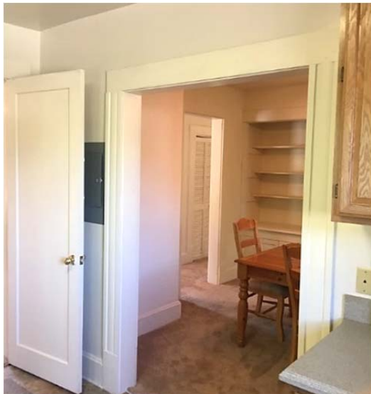
FIGURE 76. View from the lower unit kitchen to the dining room through cased openings created in the 1993 rehabilitation.
