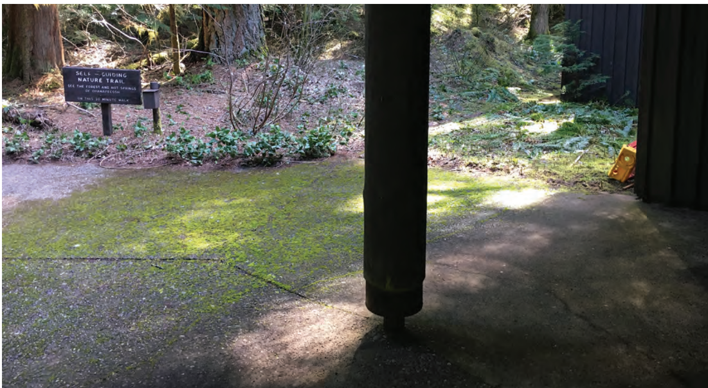
Figure 59. Care should be taken to select path and walkway surfaces that are not slippery in the campground's damp climate. The concrete aggregate around the visitor center (seen here) is very slippery. Source: NPS.
