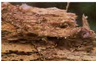
Figure 6. Laminated and pitted decayed wood with red-brown fuzzy fungal growth.
